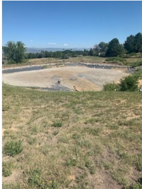
Pond 8: Empty Due to Liner Failure
