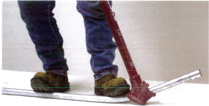
Figure 2-7. A bend with a hickey is fabricated by making several short bends at different locations along the conduit.
