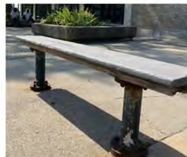
Degraded Benches at East Peterboro
