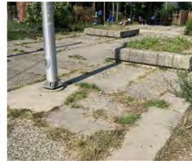
Poor Pavement Condition at West Peterboro (Typ.)
