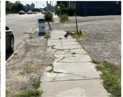
Poor Pavement Condition at Mid-block (Typ.)
