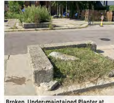
Broken, Under-maintained Planter at West Peterboro (Typ.)
