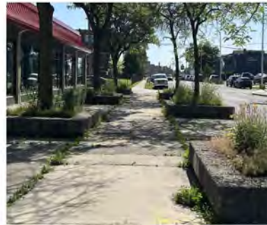
Fair to Poor Pavement Condition at East Peterboro (Typ.)
