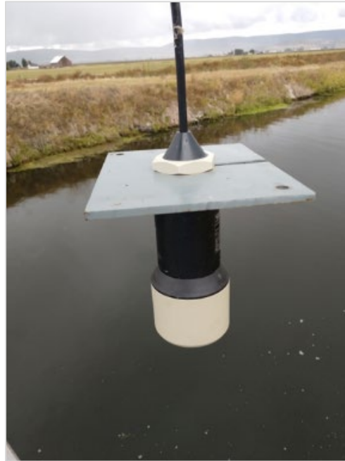
Figure 5-5. A radar sensor that reads the elevation of the water level and communicates that to the control unit.
