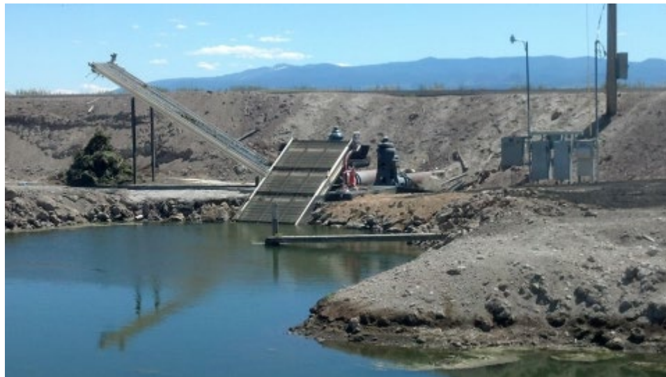
Figure 5-6. A traveling screen sits immediately upstream of the pump intake.
