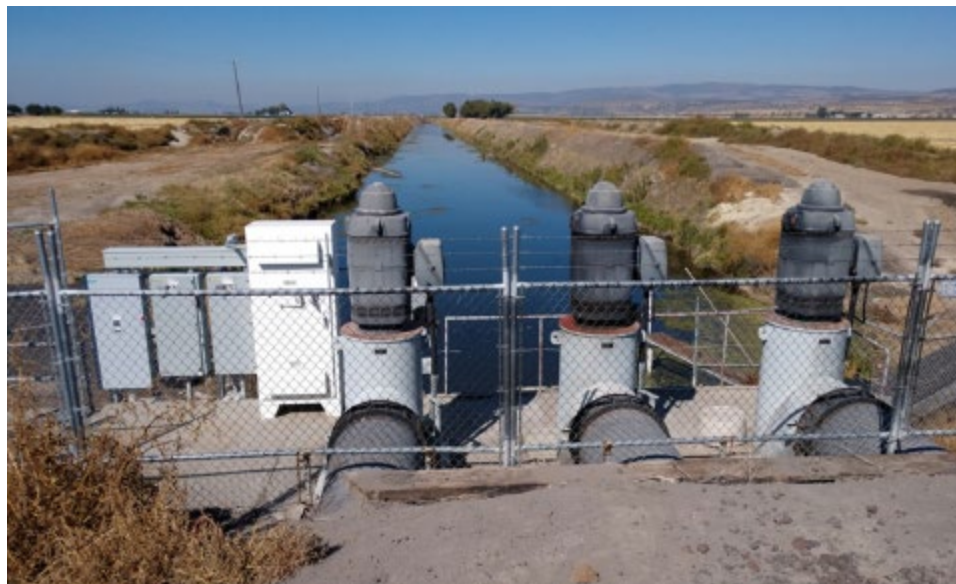
Figure 5-8. Pump site with new motors and drives.
