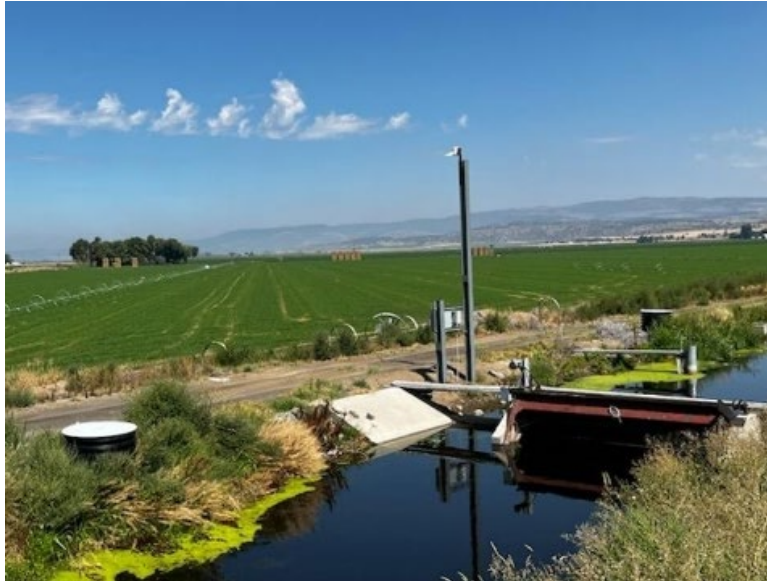
Figure 5-4. A SCADA-equipped check structure.
