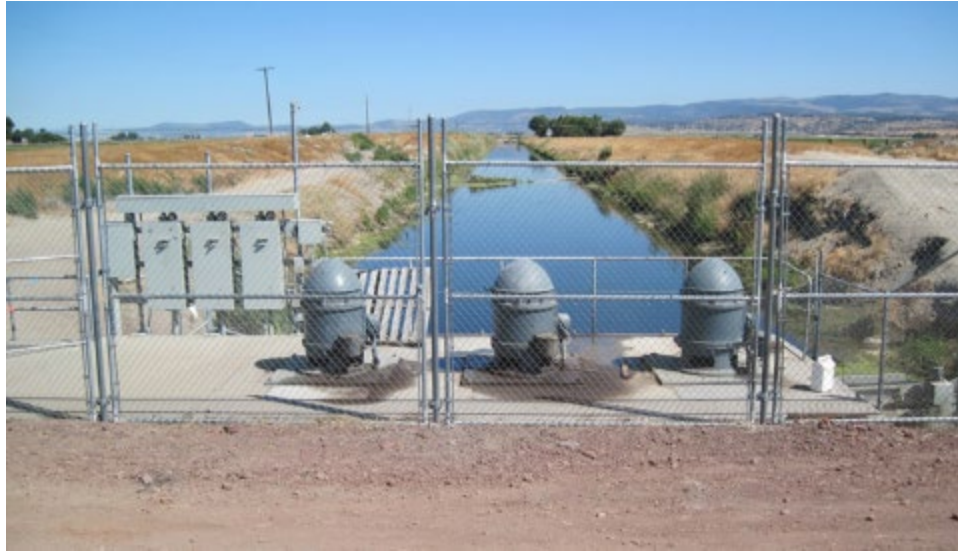
Figure 5-7. Pump site with old motors and drives.
