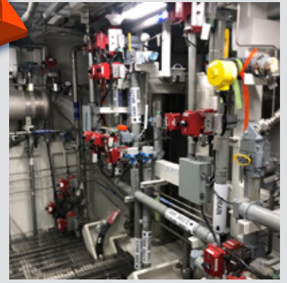
Typical field instrumentation, control wiring, and elements
