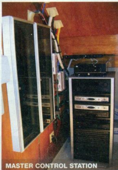
MASTER CONTROL STATION
