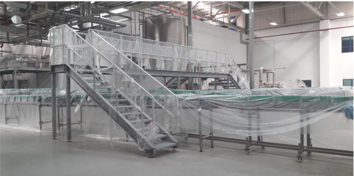
CROSSING CONVEYOR WITH STAIR AND HANDRAIL
