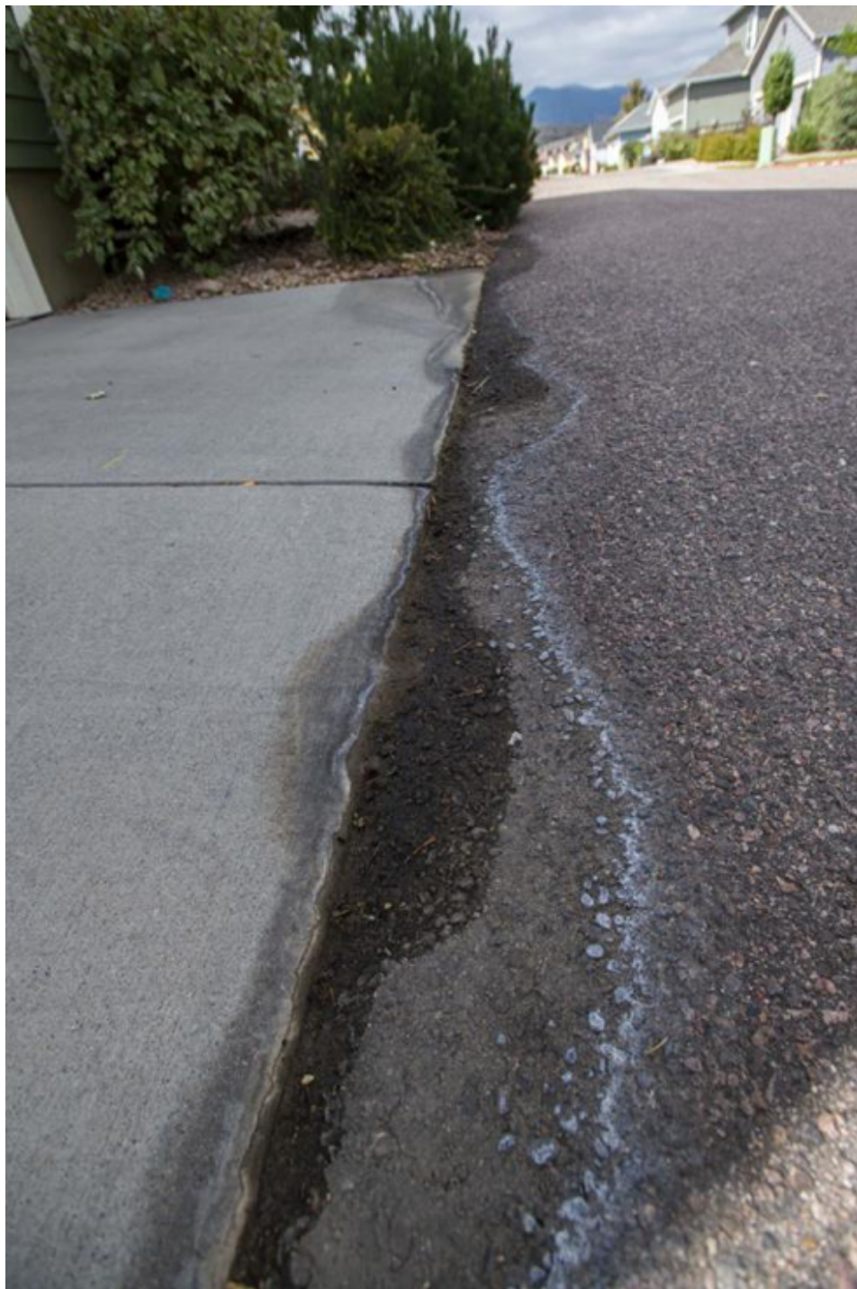
Water stains the driveway and pavement outside a home in the Gold Hill Mesa Thursday, Oct. 3, 2019. (The Gazette, Christian Murdock) CHRISTIAN MURDOCK/THE GAZETTE
