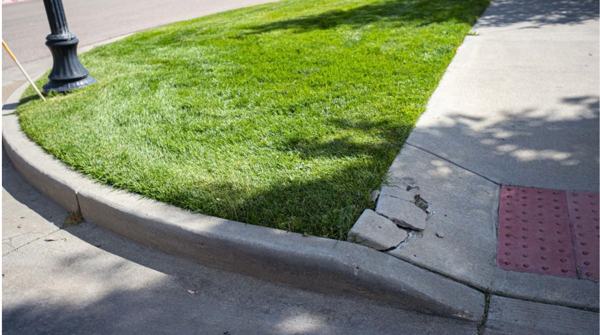
A sidewalk in the Gold Hill Mesa is cracked
