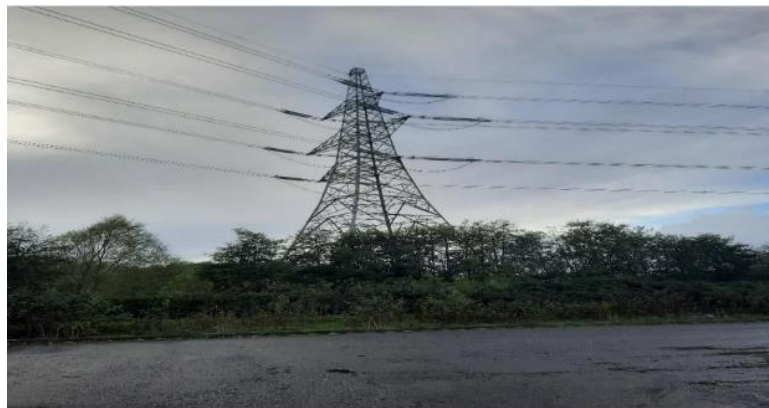
Eastern Elevation HV Pylons.
