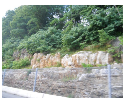
Rock Slide area on I-40
