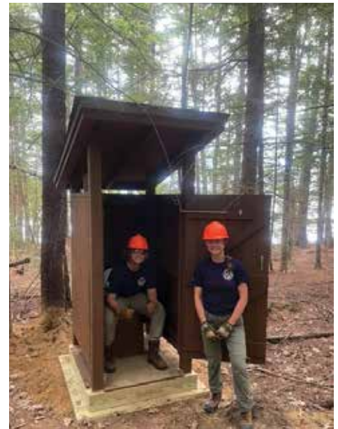
Maine Conservation Corps install privies at Downeast Land Lake Trusts water trail campsites. DLLT photo
