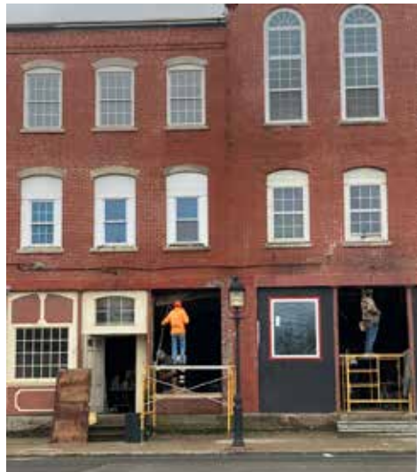
Workers continue to work steady on the facade of 449 Main Street, Calais. It is a big job, but the entire building will be renovated
