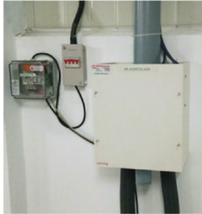
Air Switch Diverter Unit
