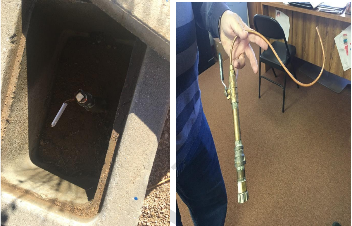
Figure 3A (left): Pipe stub in distribution system for sample collection, Figure 3B (right): S-shaped copper tool
