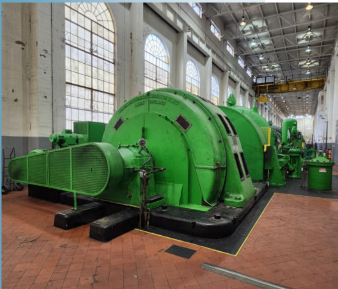
Turbine-generators at Deer Lake Power The British Thomson-Houston Co Ltd. Rugby England
