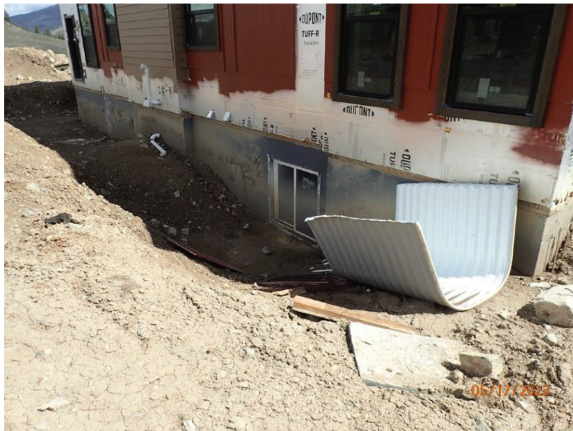
May 17, 2023, Disc OBS1, Photograph 29, DLC, 101 Mule Deer Court, backfilling along west elevation.
