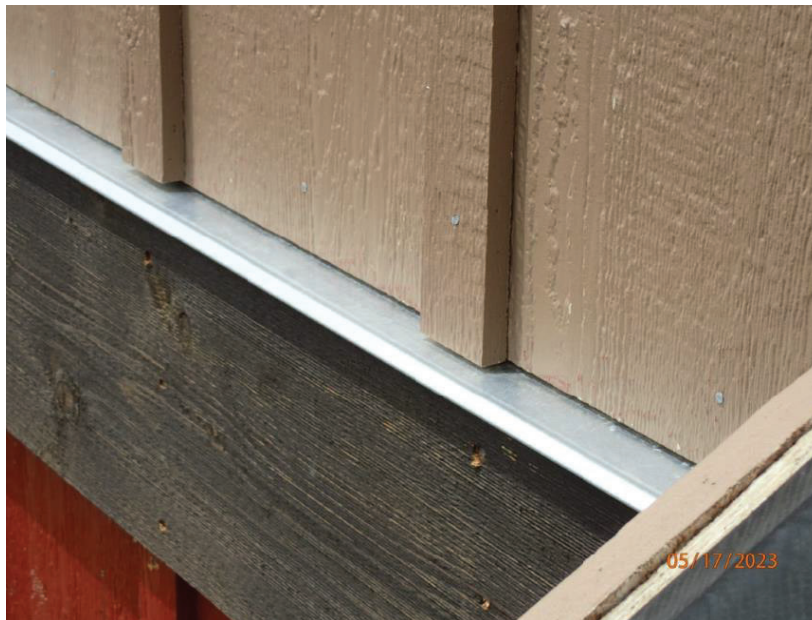
May 17, 2023, Disc OBS1, Photograph 310, DLC, 101 Mule Deer Court, non-compliant clearance between siding and thru-wall flashing. Flashing also installed flat, minimum of five-degree slope is required.
