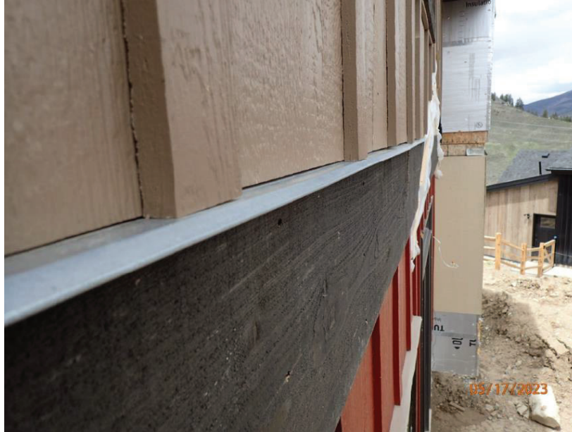
May 17, 2023, Disc OBS1, Photograph 273, DLC, 101 Mule Deer Court, non-compliant clearance between siding and thru-wall flashing. Flashing also installed flat, minimum of five-degree slope is required.
