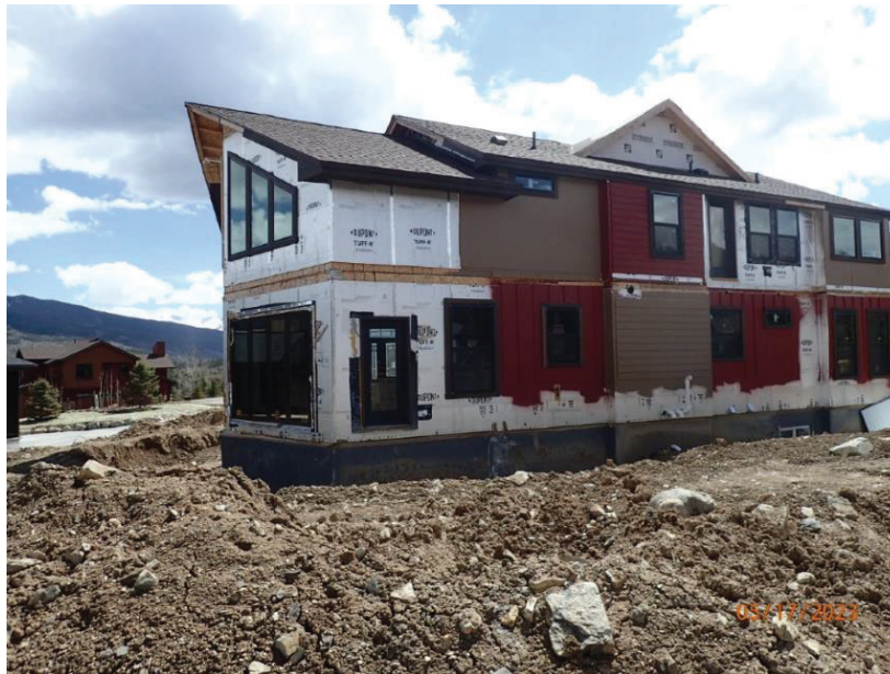
May 17, 2023, Disc OBS1, Photograph 9, DLC, 101 Mule Deer Court, spoil materials piled without a swale to direct water off the site.
