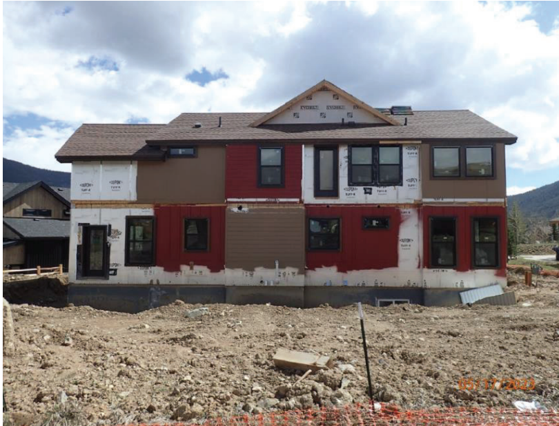
May 17, 2023, Disc OBS1, Photograph 8, DLC, 101 Mule Deer Court, incomplete exterior siding installation at west elevation.
