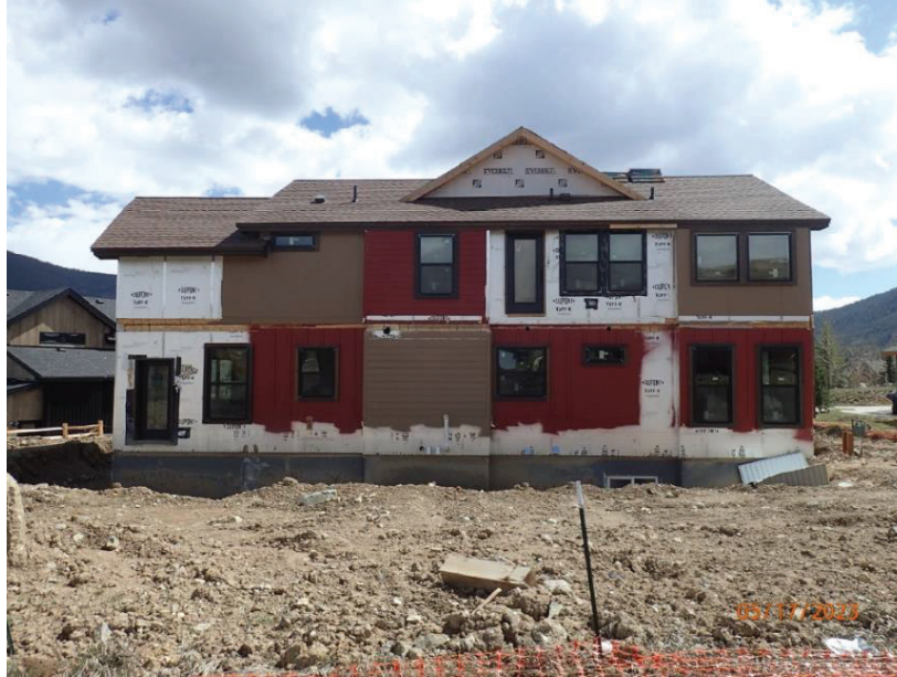
May 17, 2023, Disc OBS1, Photograph 8, DLC, 101 Mule Deer Court, spoil materials piled without a swale to direct water off the site.
