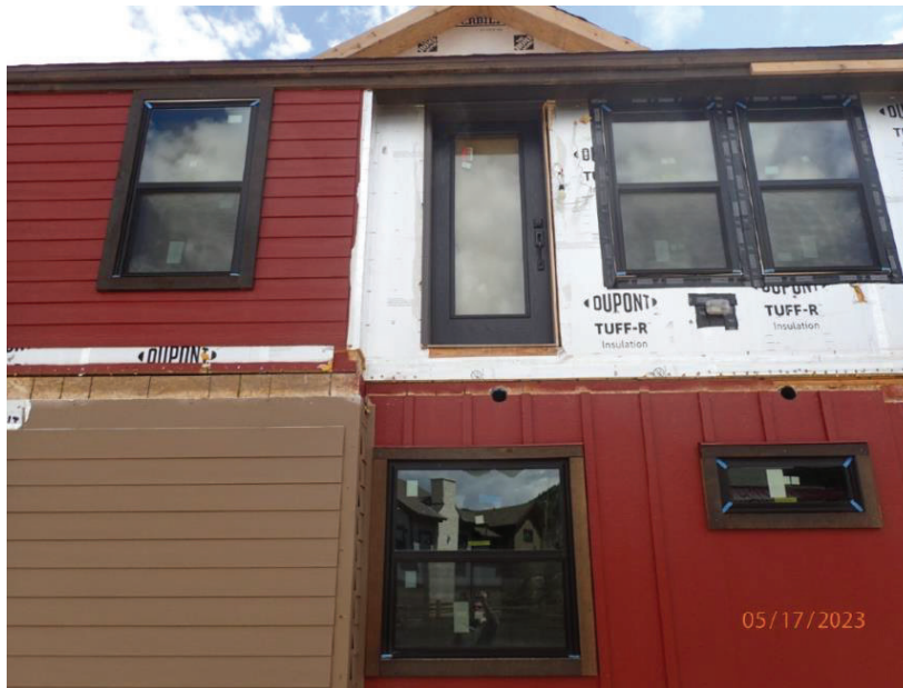
May 17, 2023, Disc OSB1, Photograph 35, DLC, 101 Mule Deer Court, exterior deck not constructed and incomplete siding installation on west elevation.
