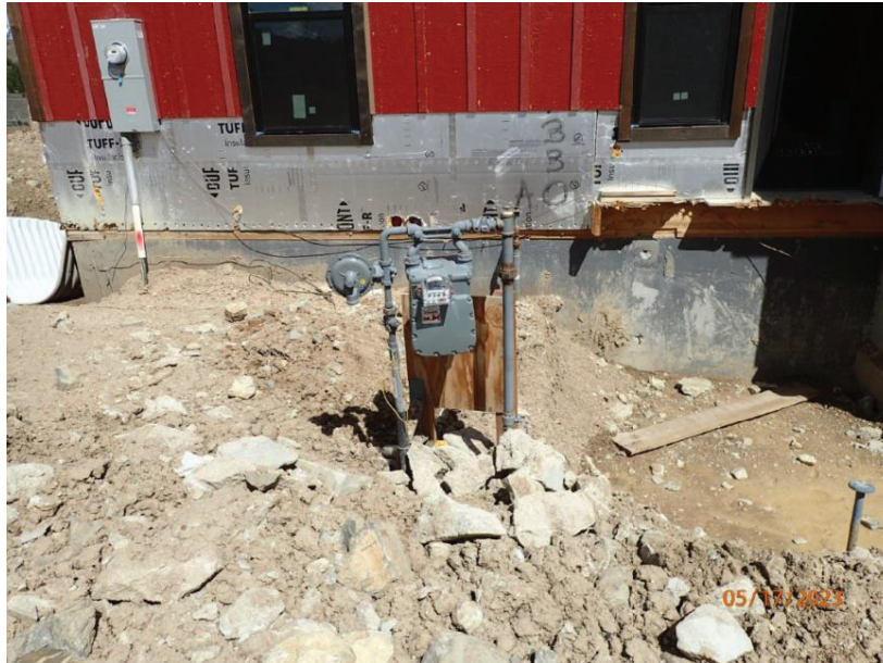
May 17, 2023, Disc OBS1, Photograph 23, DLC, 101 Mule Deer Court, improper backfill and poor support of gas meter and line at south elevation.
