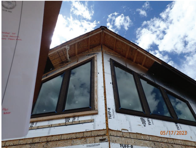
May 17, 2023, Disc OBS1, Photograph 50, DLC, 101 Mule Deer Court, missing soffit.
