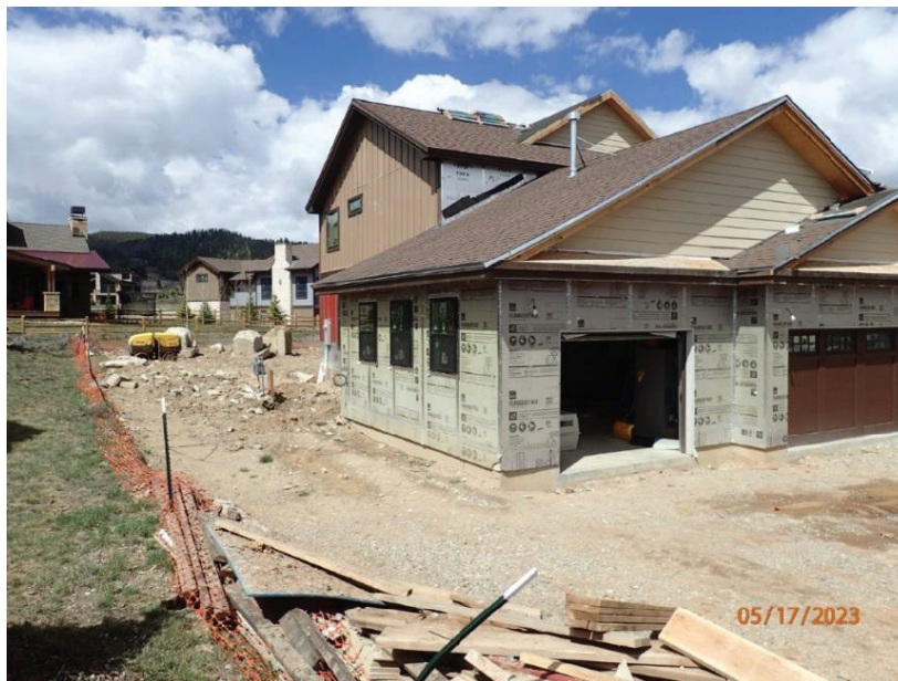
May 17, 2023, Disc OBS1, Photograph 4, DLC, 101 Mule Deer Court, no drainage swale in place to direct water away from the foundation.
