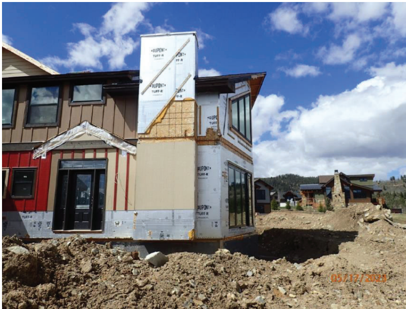
May 17, 2023, Disc OBS1, Photograph 12, DLC, 101 Mule Deer Court, spoil materials piled without a swale to direct water off the site.
