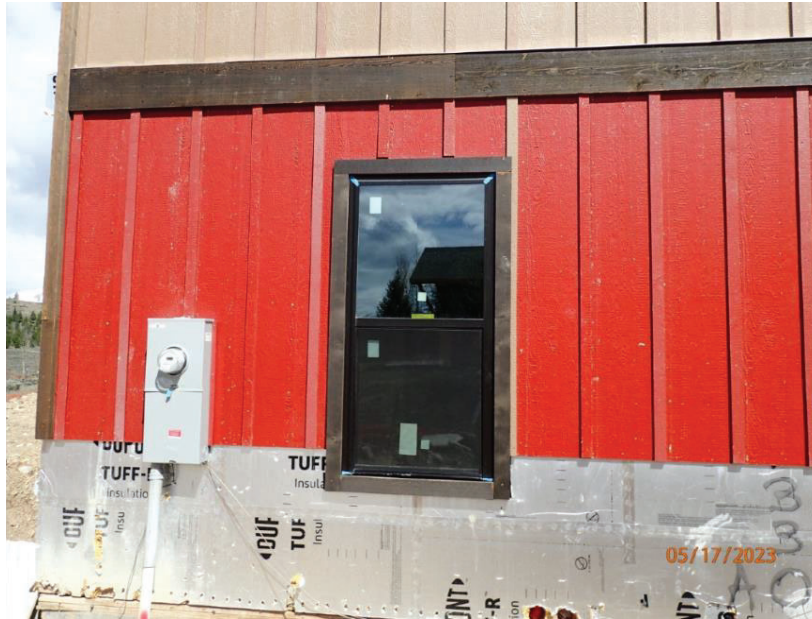
May 17, 2023, Disc OBS1, Photograph 26, DLC, 101 Mule Deer Court, incomplete exterior finish installation at south elevation.
