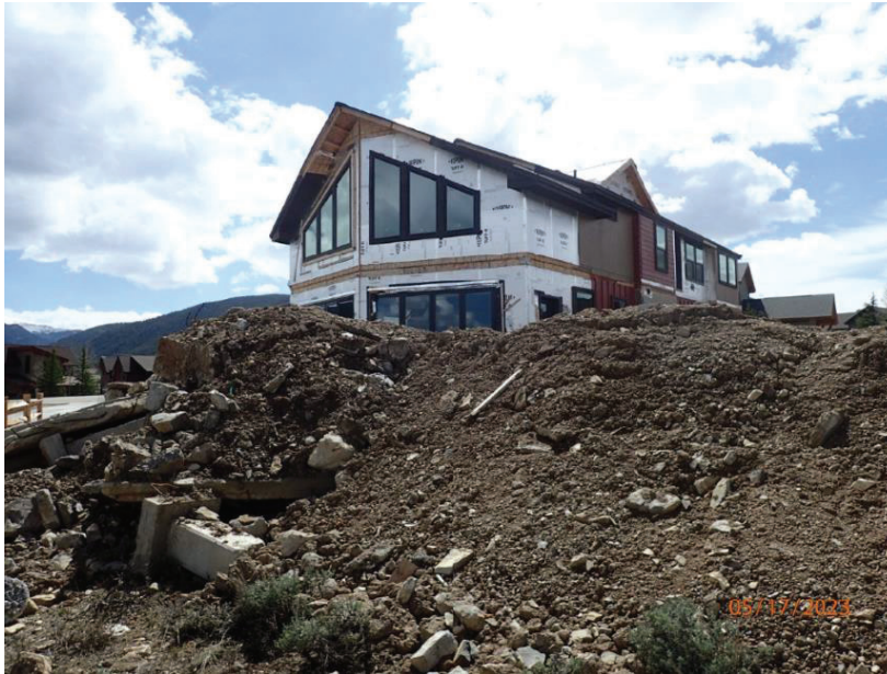
May 17, 2023, Disc OBS1, Photograph 10, DLC, 101 Mule Deer Court, spoil materials piled without a swale to direct water off the site.
