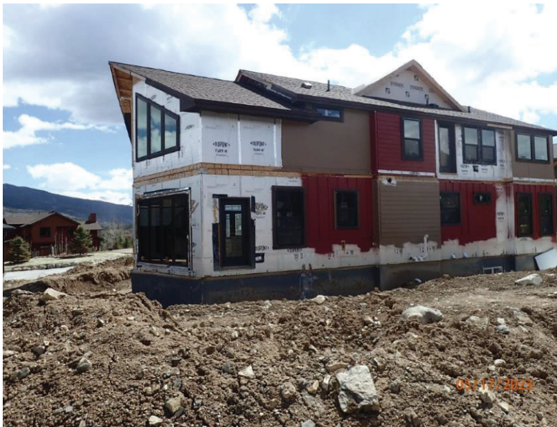
May 17, 2023, Disc OBS1, Photograph 9, DLC, 101 Mule Deer Court, incomplete siding installation at northeast elevation.
