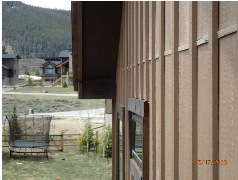
May 17, 2023, Disc OBS1, Photograph 312, DLC, 101 Mule Deer Court, missing head flashing at window.
