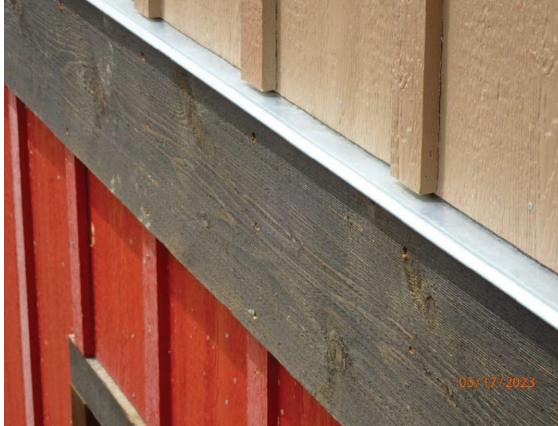
May 17, 2023, Disc OBS1, Photograph 311, DLC, 101 Mule Deer Court, non-compliant clearance between siding and thru-wall flashing. Flashing also installed flat, minimum of five-degree slope is required.
