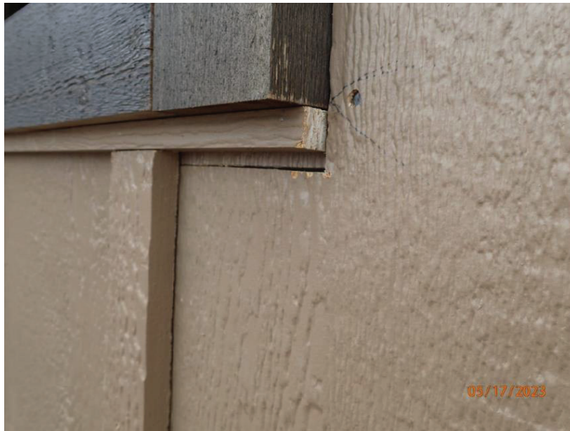
May 17, 2023, Disc OBS1, Photograph 280, DLC, 101 Mule Deer Court, untreated cut ends and short cut siding below upper level windows. The small piece of trim is used to fill to undercut panel below the window.
