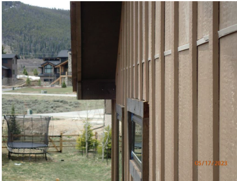
May 17, 2023, Disc OBS1, Photograph 312, DLC, 101 Mule Deer Court, missing flashing at window head and non-compliant thru-wall flashing between horizontal joint in vertical panel siding.
