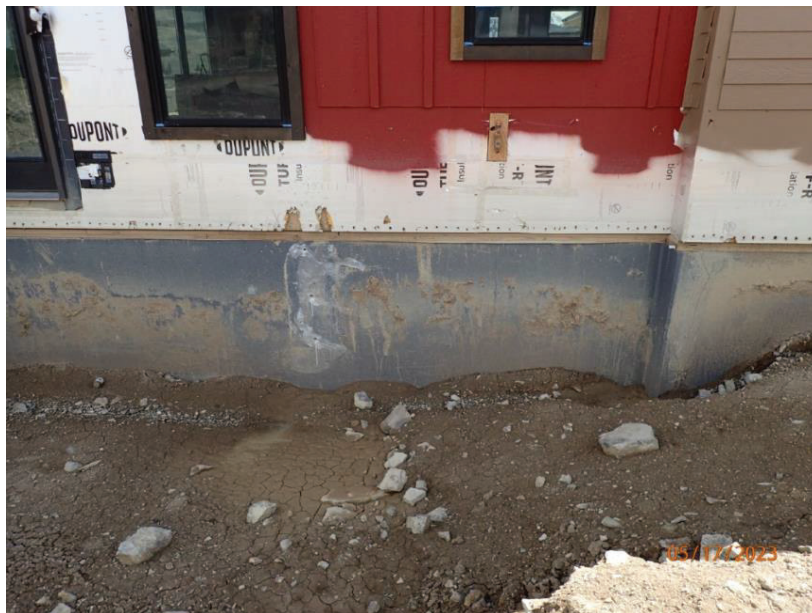
May 17, 2023, Disc OBS1, Photograph 37, DLC, 101 Mule Deer Court, backfilling along west elevation.
