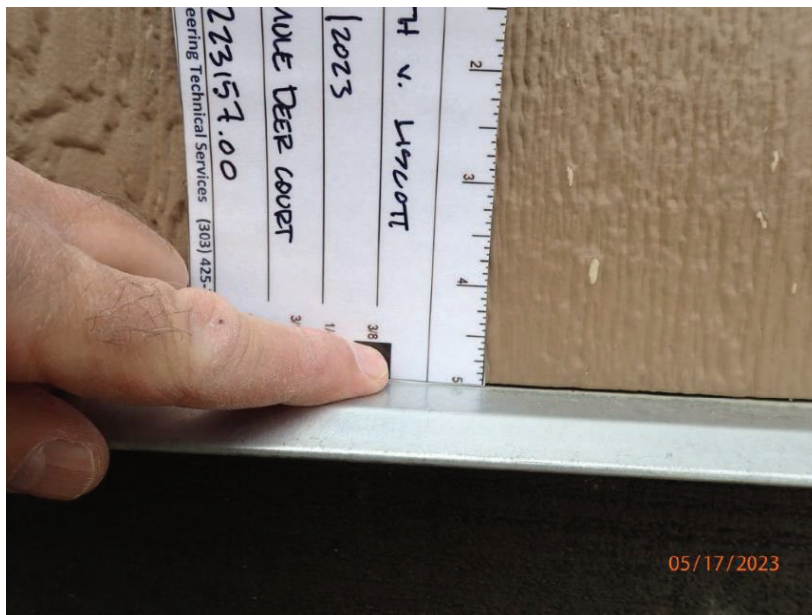
May 17, 2023, Disc OBS1, Photograph 272, DLC, 101 Mule Deer Court, non-compliant clearance between siding and thru-wall flashing. Flashing also installed flat.
