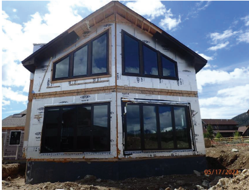
May 17, 2023, Disc OBS1, Photograph 11, DLC, 101 Mule Deer Court, incomplete siding installation at north elevation.
