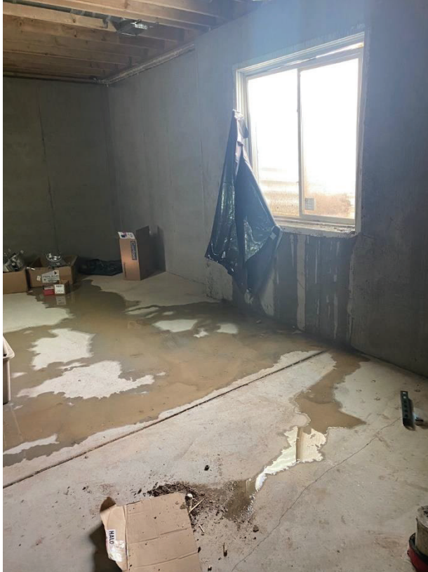
Owner provided photo showing water coming through the basement window.
