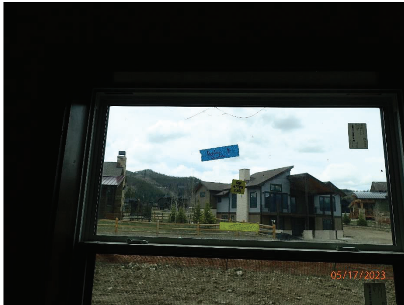
May 17, 2023, Disc OBS1, Photograph 319, DLC, 101 Mule Deer Court, broken window at first floor bath.
