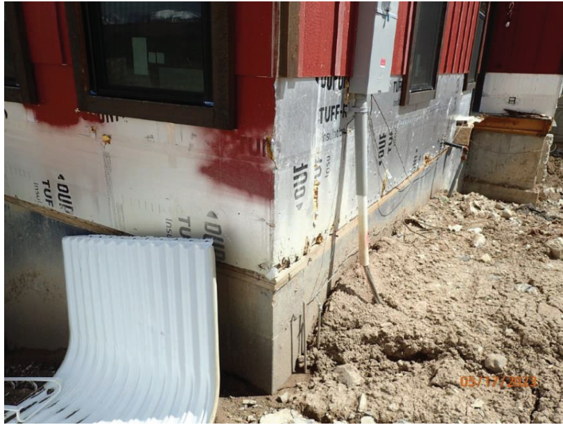
May 17, 2023, Disc OBS1, Photograph 31, DLC, 101 Mule Deer Court, improper backfill at southwest corner of structure.
