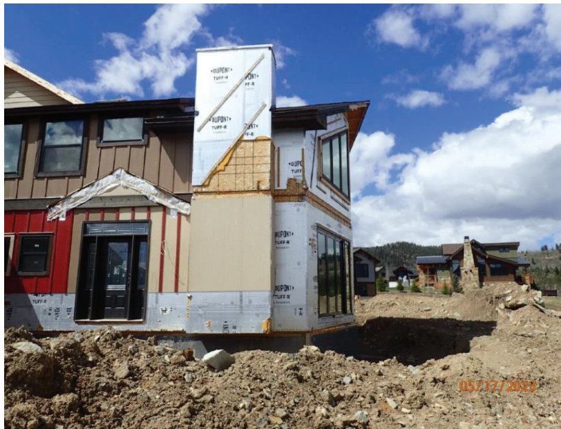
May 17, 2023, Disc OBS1, Photograph 12, DLC, 101 Mule Deer Court, incomplete siding installation at east elevation.
