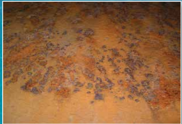
General corrosion on hull plate.
