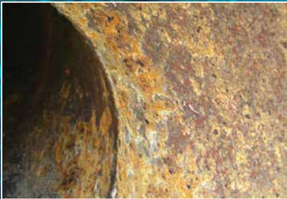
Pitting corrosion around exhaust discharge.
