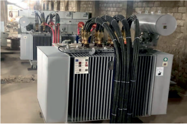
Sultan Family 6MVA Trafo Tesisi
