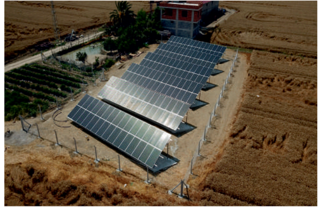
Akdemir GES / 73,8kWp
