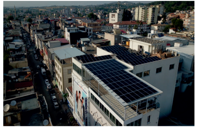
LCW GES / 76,44kWp
