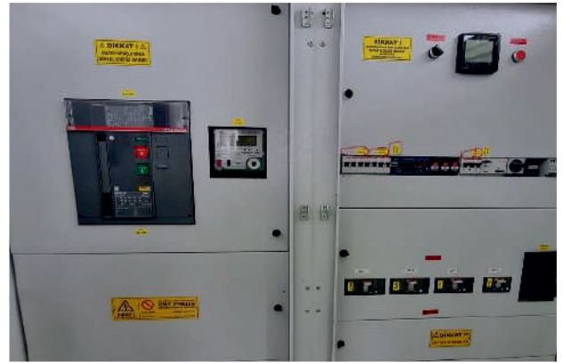
SPP Panel Measurement and Controls
