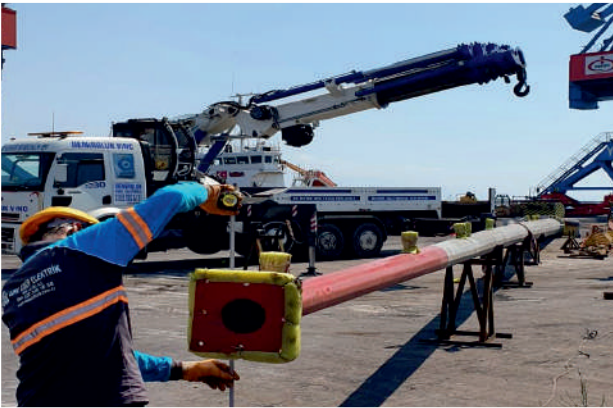
İsdemir 17 Pole Perimeter Lighting
