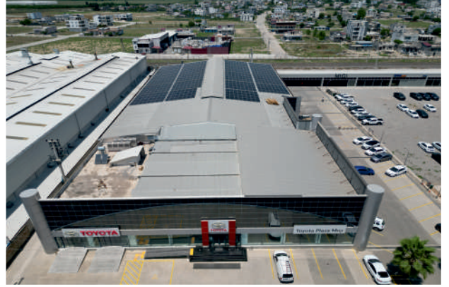
Toyota Plaza Mıçı SPP / 950kWp
