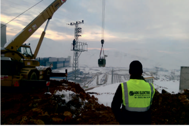
Pole Mounted Transformer
