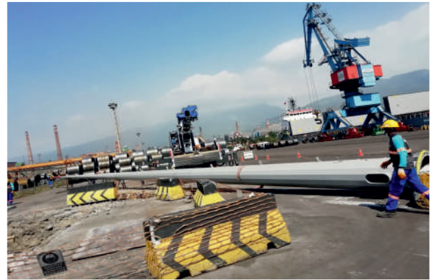
İsdemir 17 Pole Perimeter Lighting
