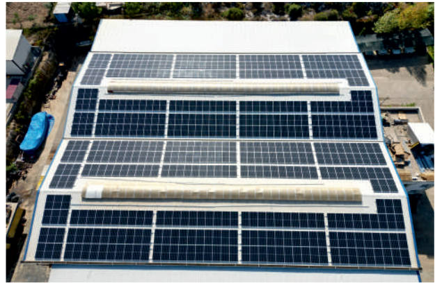
Nika SPP / 950kWp
