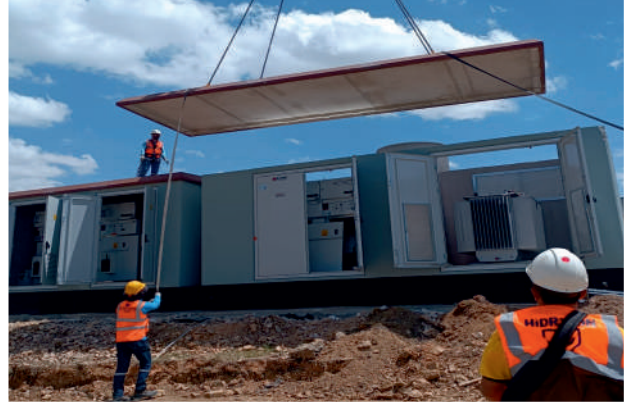
Fernas 7.5MVA Transformer Plants
