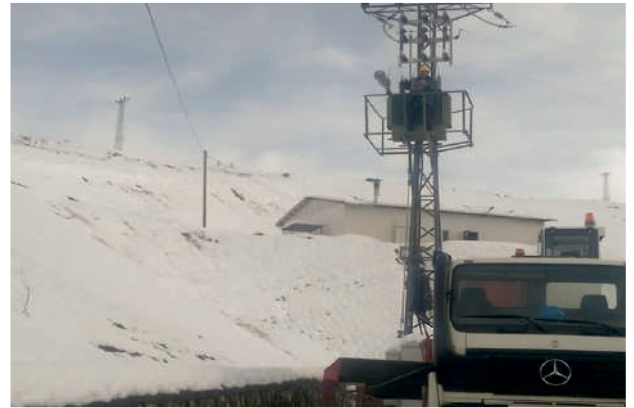
Pole Mounted Transformer
