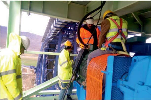
Belt Conveyor Motor Connection
