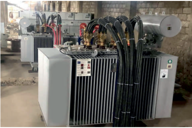
Sultan Family 6MVA Transformer Plants
