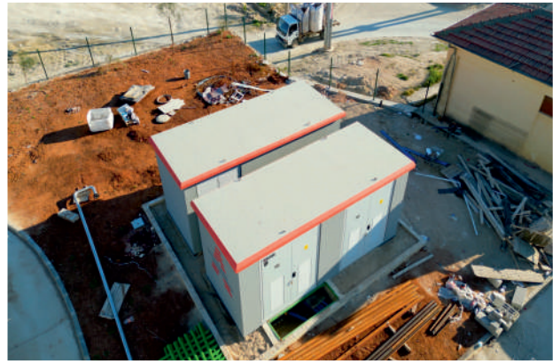
Green Enerji 1250kVA Transformer Plants
