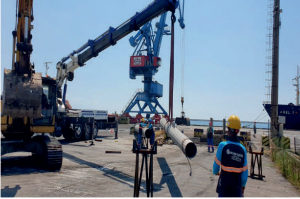
İsdemir 17 Pole Perimeter Lighting
