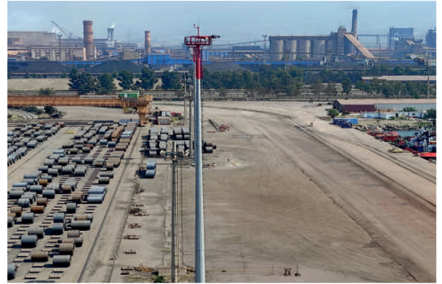
İsde mir 17 Pole Perimeter Lighting
