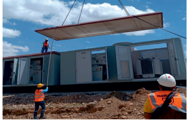
Fernas 7.5MVA Transformer Plants
