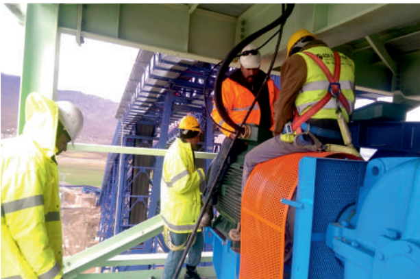
Belt Conveyor Motor Connection
