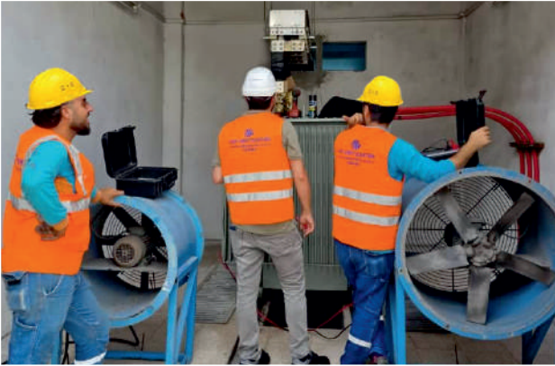
Transformer Winding Resistance and Megger Insulation Test
