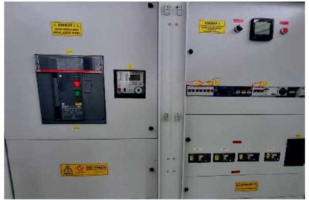
SPP Panel Measurement and Controls
