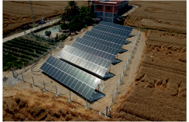
Akdemir SPP / 73,8kWp
