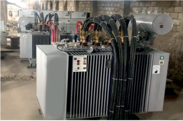
Sultan Family 6MVA Transformer Plants
