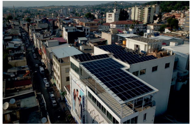
LCW SPP / 76,44kWp
