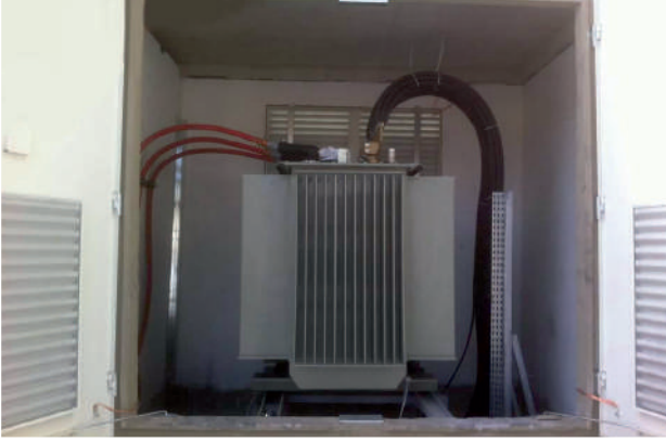
Emta 7MVA Transformer Plants
