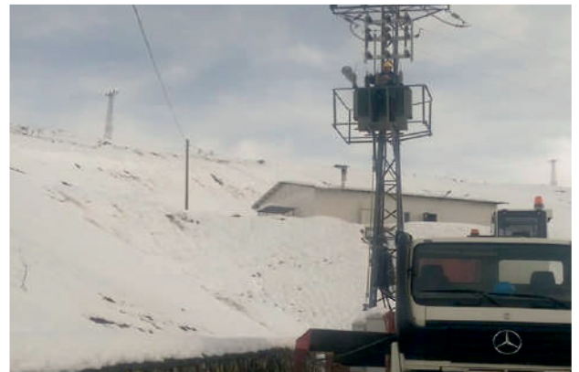
Pole Mounted Transformer
