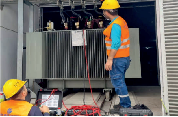
Transformer Cycle Ratio Measurements
