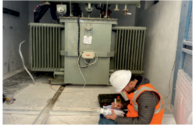
Transformer Oil Analysis
