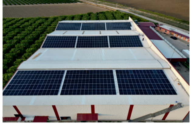
Orbaç SPP / 288,02kWp
