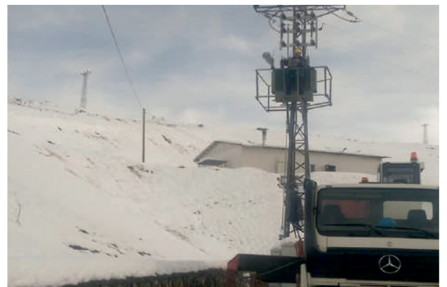
Pole Mounted Transformer
