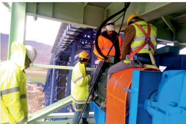
Belt Conveyor Motor Connection
