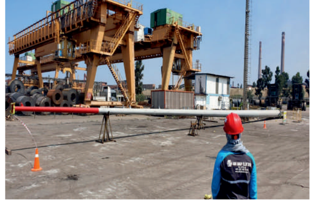
İsdemir 17 Pole Perimeter Lighting
