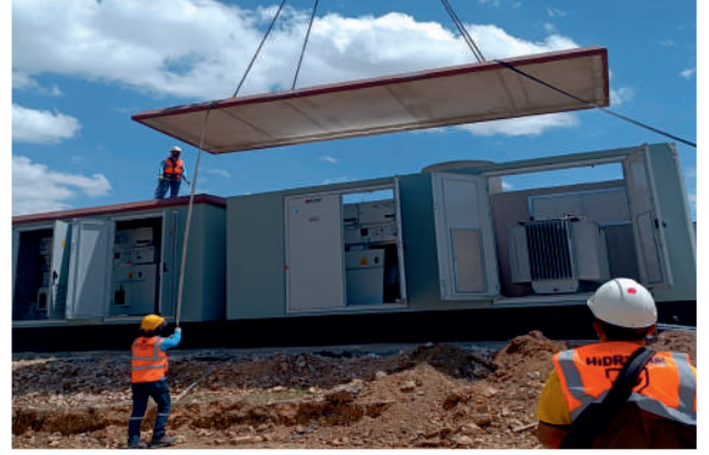
Fernas 7.5MVA Transformer Plants
