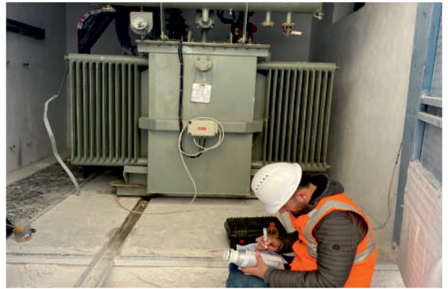
Transformer Oil Analysis
