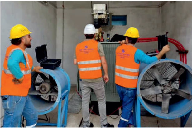
Transformer Winding Resistance and Megger Insulation Test
