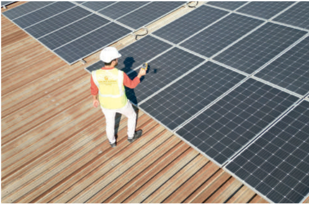
SPP Thermal Camera Controls
