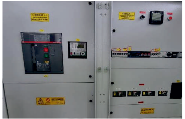
SPP Panel Measurement and Controls
