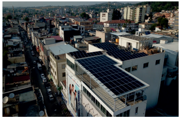
LCW SPP / 76,44kWp
