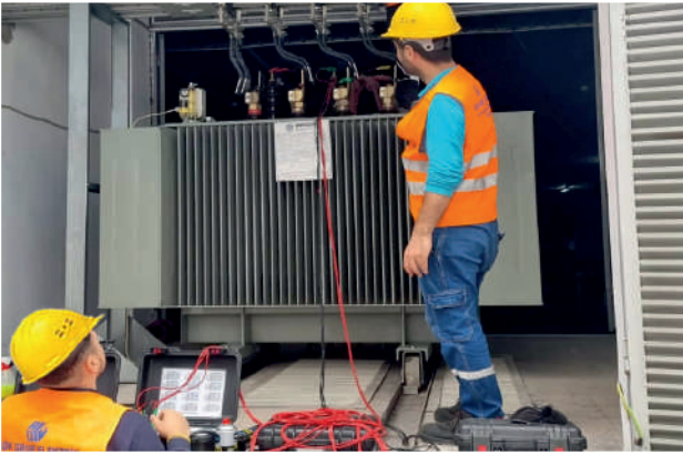
Transformer Cycle Ratio Measurements
