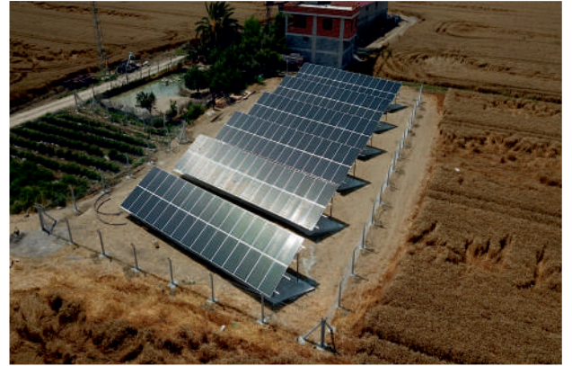
Akdemir GES / 73,8kWp
