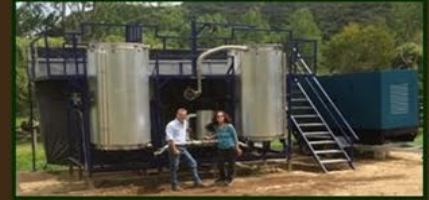
2021 - extraction plant, commissioned/ready
