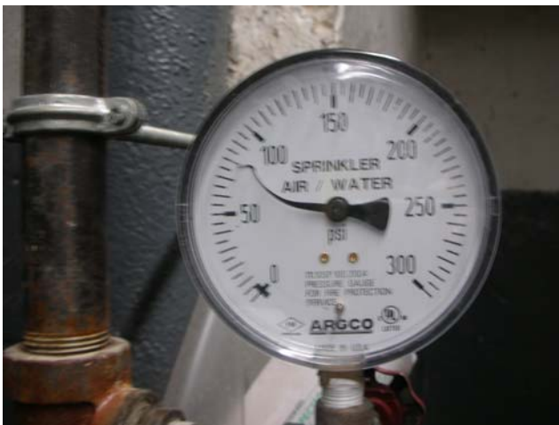
Defective Water Pressure Gauge
