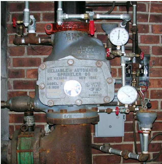
Dry Pipe Valve Assembly
