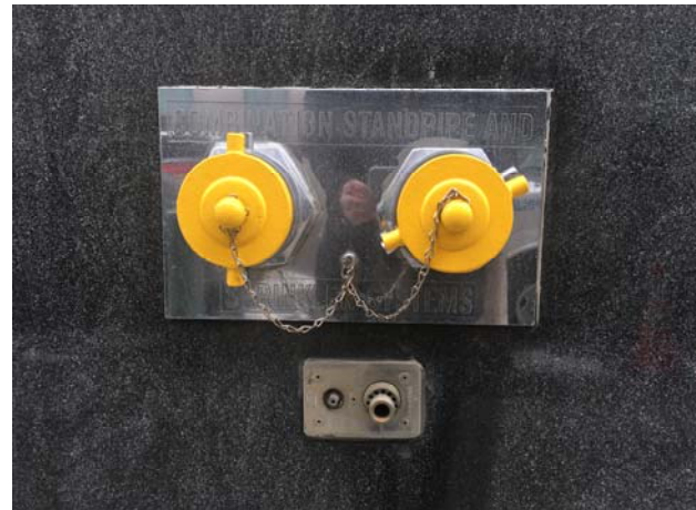
Sprinkler & Standpipe Fire Department Connections
