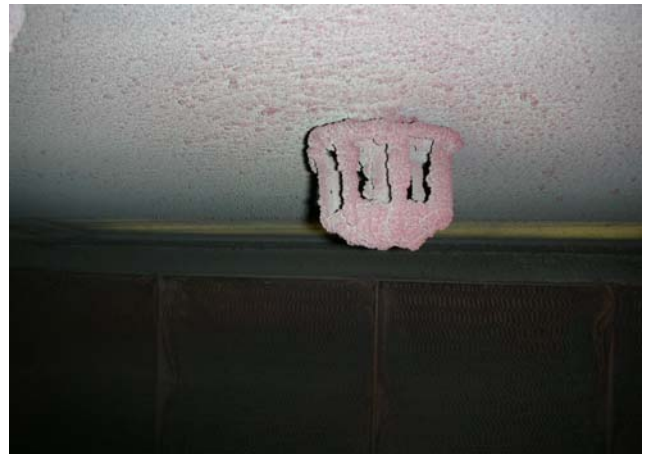
Loaded Sprinkler in Head Cage Head
