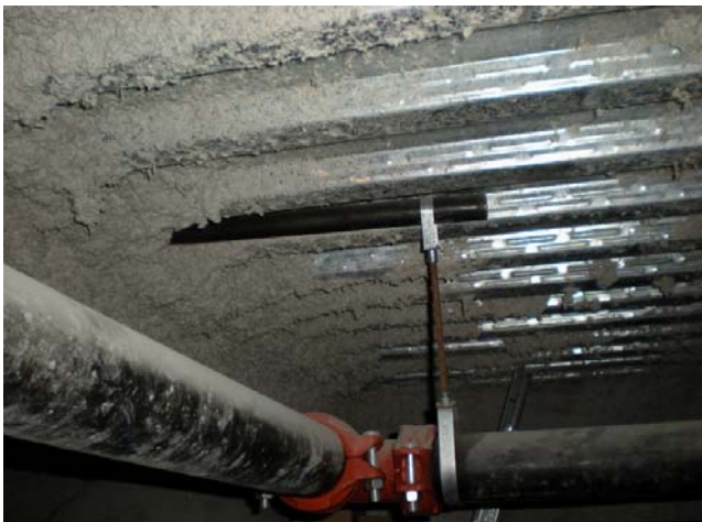
Sprinkler System Improper Hanger
