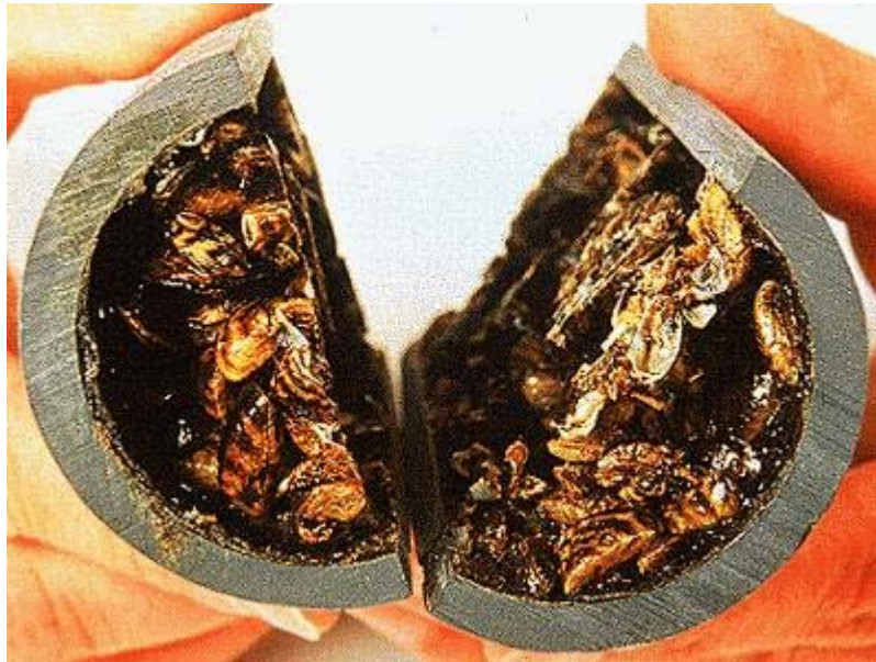
Piping Infested with Zebra Mussels
