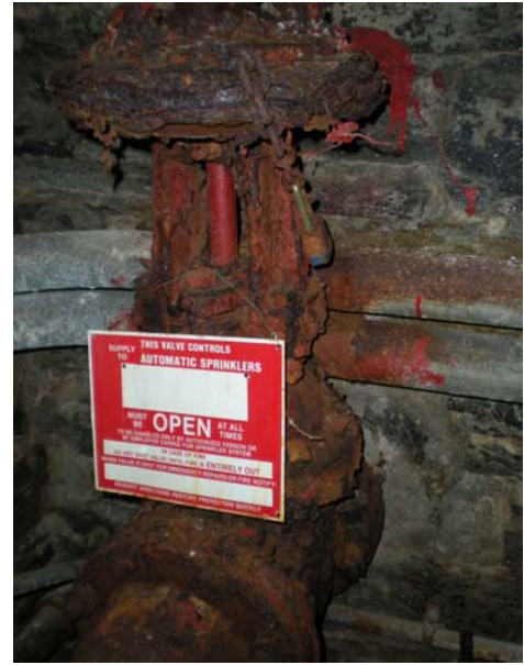
Corroded Curb Valve in Sidewalk Vault
