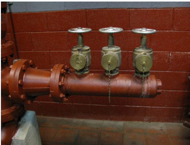
Fire Department Test Manifold
