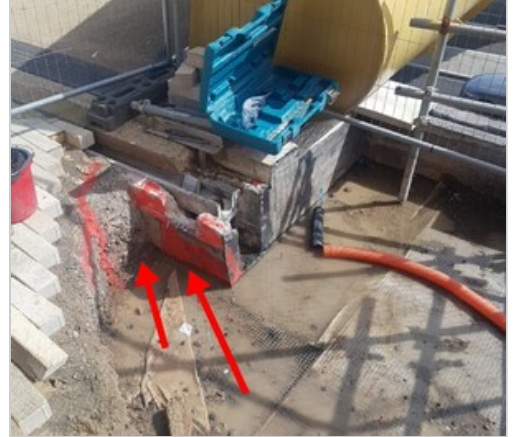
Highlighted by red to be broke, exposed and repairs
