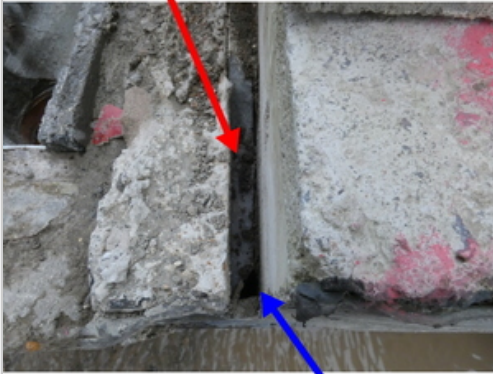
Water test aprox 6 liter - 04.04.23
