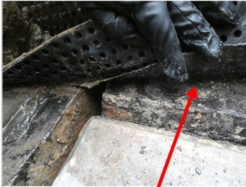
Membrane not stick to concrete
