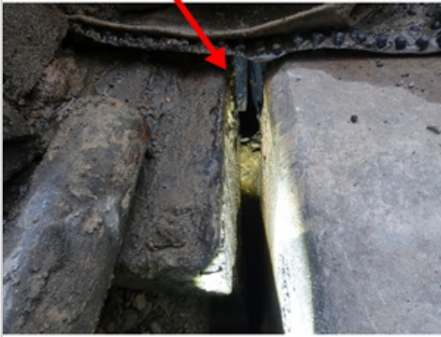
4 Missing Weatherproof Membrane and Concrete Seal
