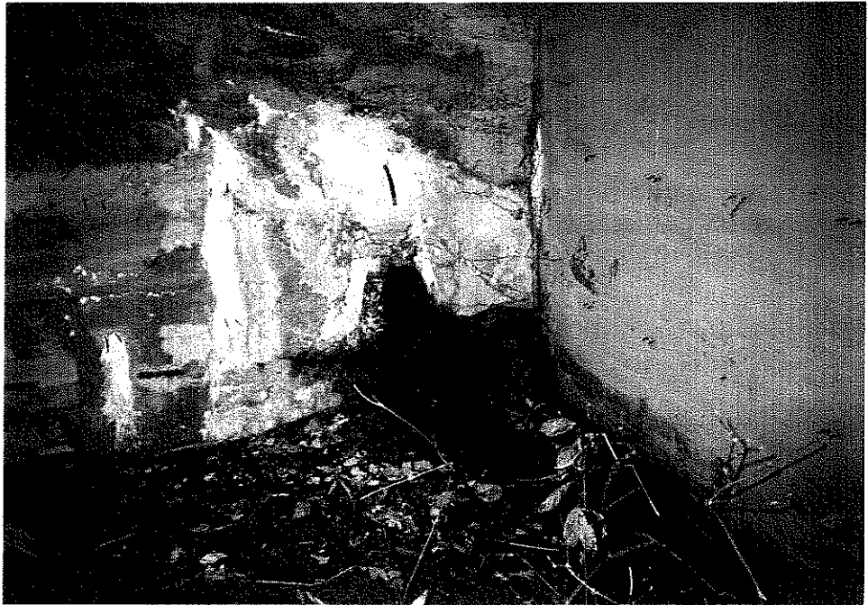
PHOTO #5 SEEPAGE OF WATER THROUGH DAM, SOUTH OF CREEK
