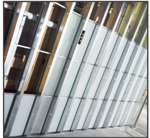
ASRP lead plates installed before drywall. Our system features clean, straight lines.
