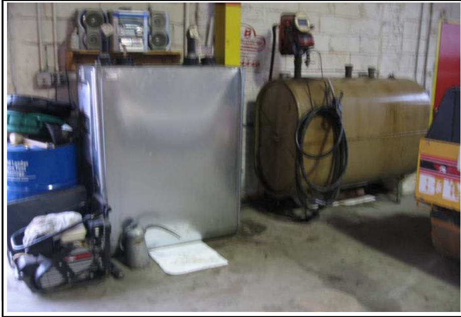
Photo No.: 55 Date: 12/11/2008 Description: View of two 275-gallon fuel oil ASTs (AOC 1) located within Building K.
