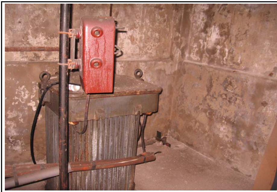
Photo No.: 34 Date: 12/11/2008 Description: View of pad-mounted transformer (AOC 5) located in Building A.
