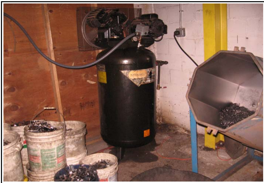
Photo No.: 24 Date: 12/11/2008 Description: View of air compressor unit (AOC 15) and finished gun holster clips located in Building M1.
