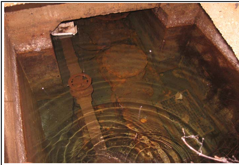
Photo No.: 38 Date: 12/11/2008
