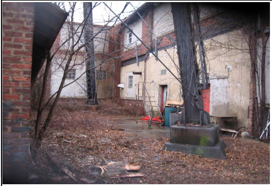
Photo No.: 41 Date: 12/11/2008
