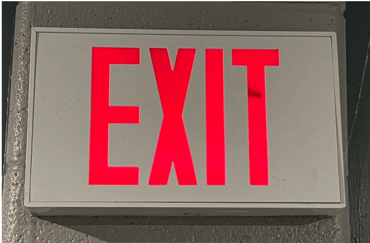
An example of a standalone exit sign.
