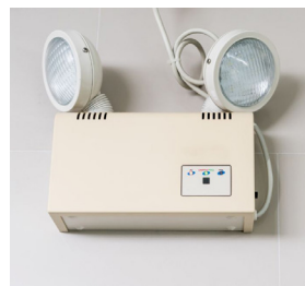
An example of a power pack emergency light.
