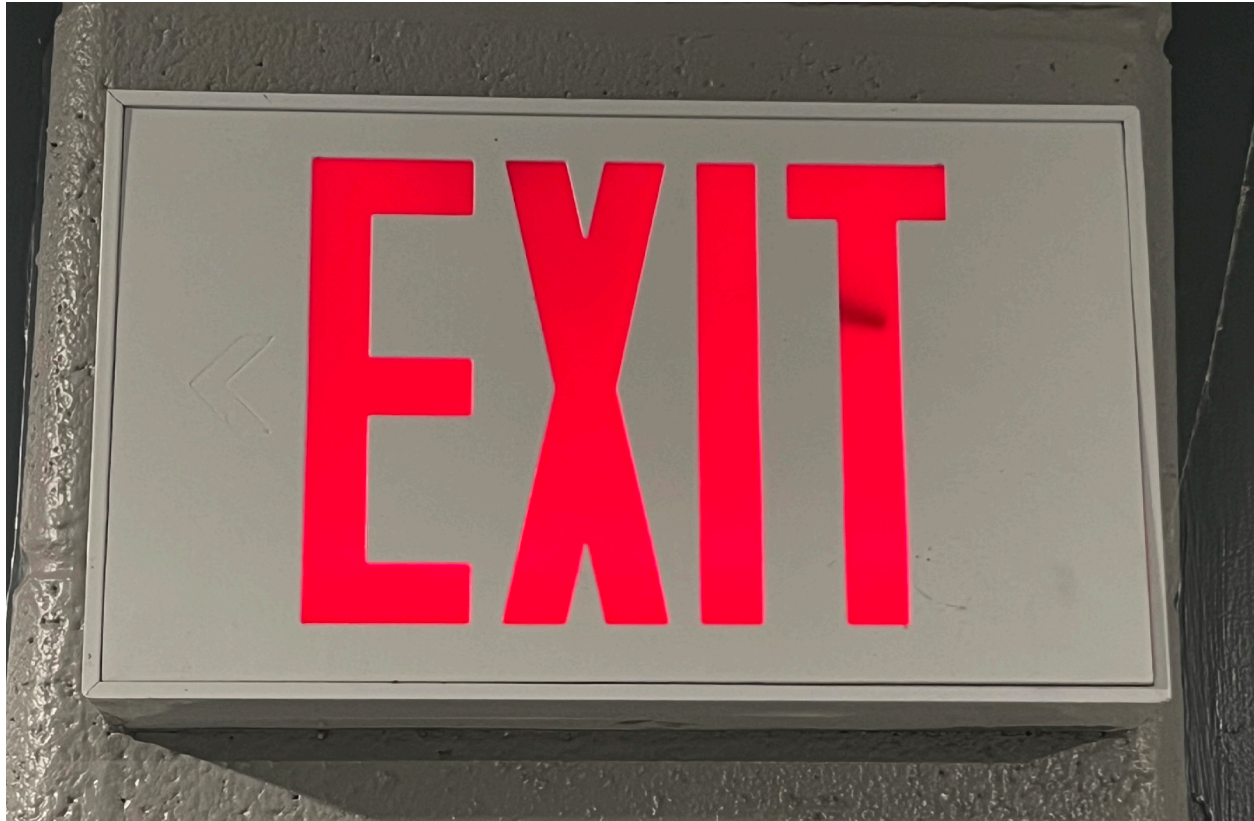
An example of a standalone exit sign.
