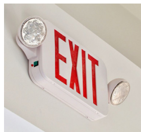
An example of an emergency light combination unit.
