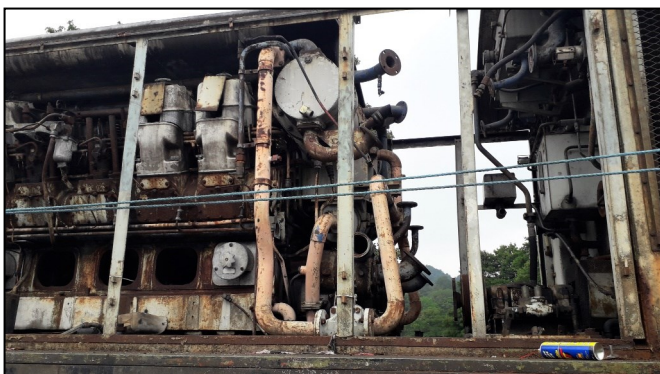
The connections to the cooler group have been removed. This space is also where the compressors – long since removed – would have been.
