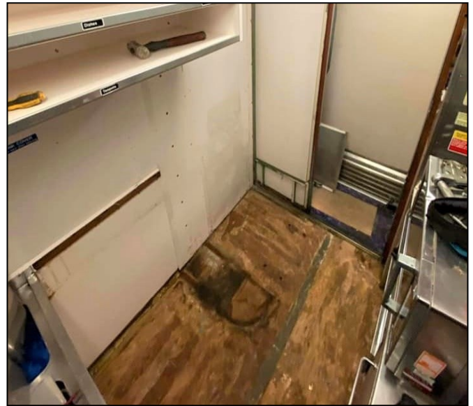
The old flooring has been removed and some cupboards taken out to make space for the water heater.
