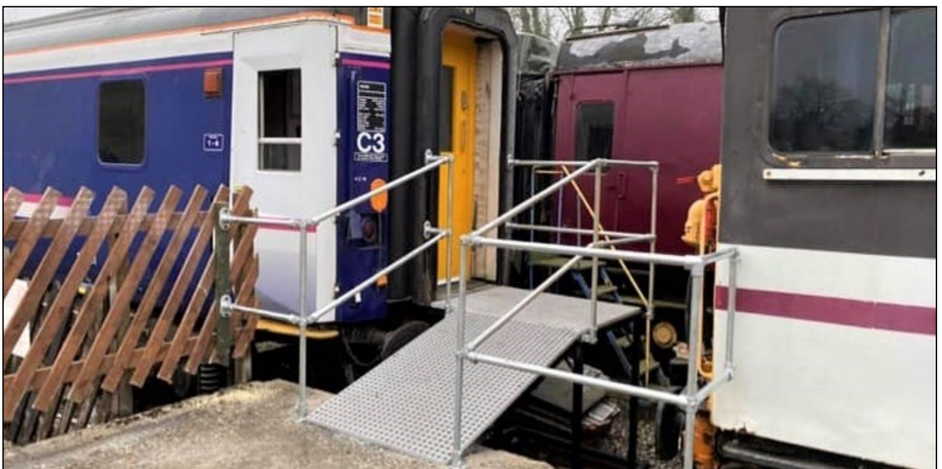
The finished access ramp in place and ready for the first residents.
