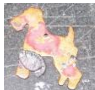
#13 Take flaking Scalex coating off, then clean.
