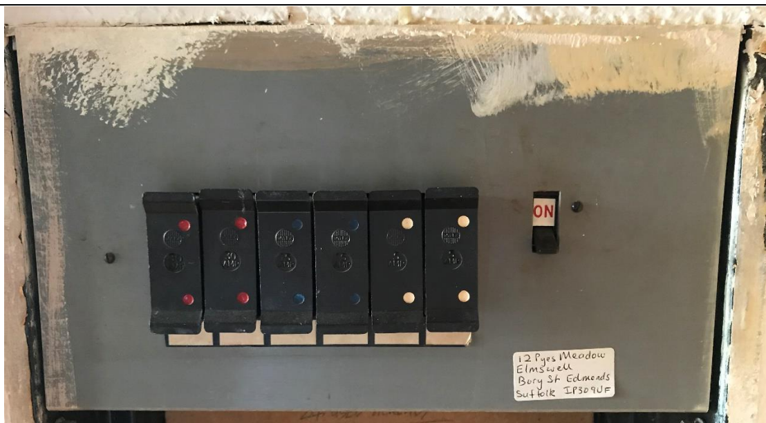
(1) Wylex 'M Series 60 Range' Rewireable BS3036 Skeleton Fuseboard c/w rewirable fuses
