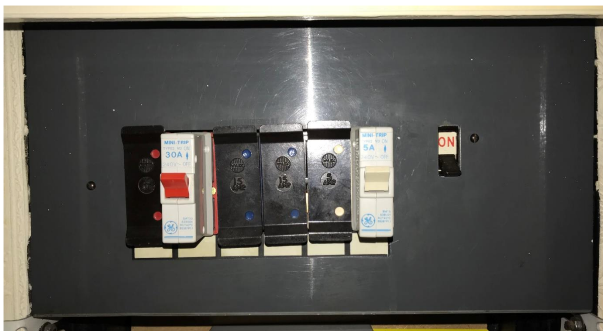
(1) Wylex 'M Series 60 Range' Rewireable BS3036 Skeleton Fuseboard c/w rewirable fuses and miniature circuit breakers (MCB)
