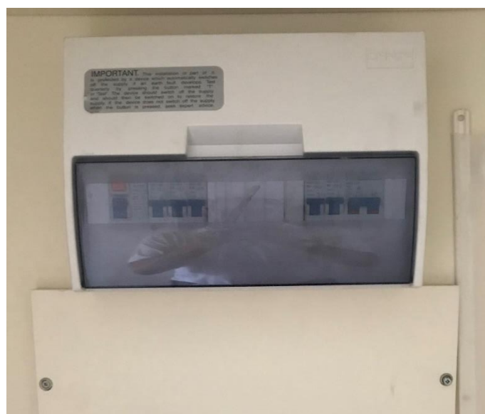
(2) Modern plastic Split load consumer unit c/w MCB and one Residual Current Device (RCD) Main Switch
