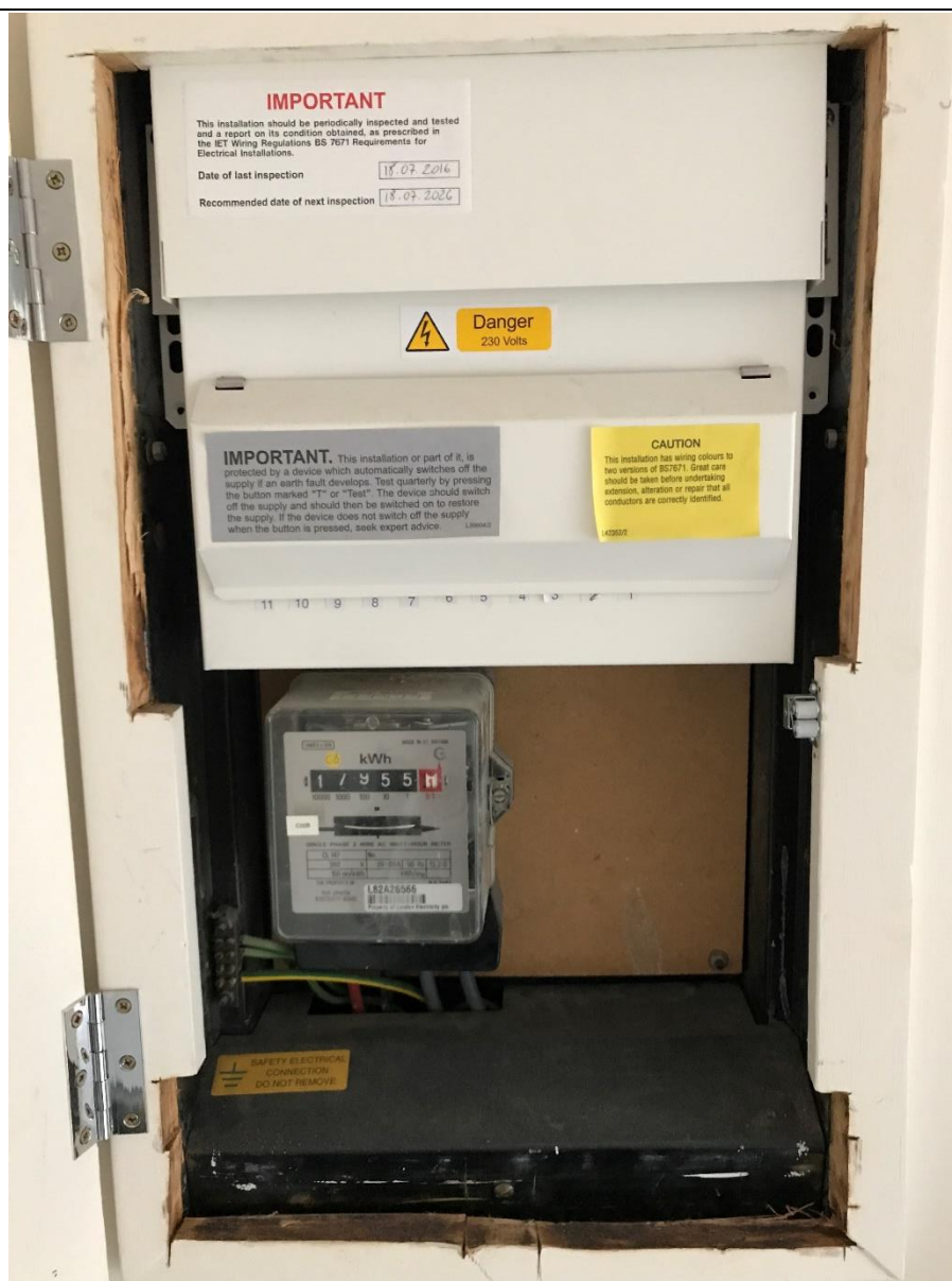
(4) Wylex metal cased split load consumer unit, dual RCD protection to all MCB circuits.
