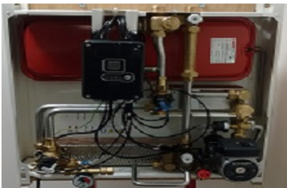
Figure 1 Heat Interface Unit
