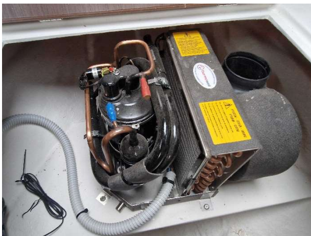
Air condition unit
