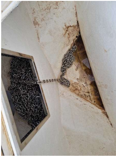
Chain locker and anchor chain
