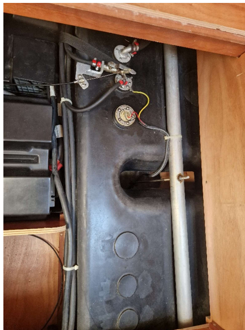
Diesel oil tanks
