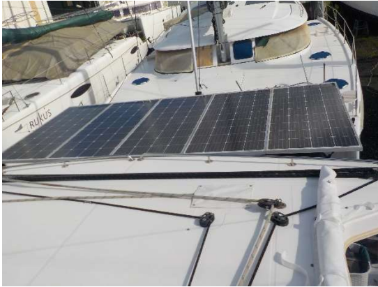
Five Solar Panels, 175w each
