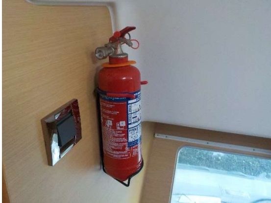
Fire extinguisher port aft cabin
