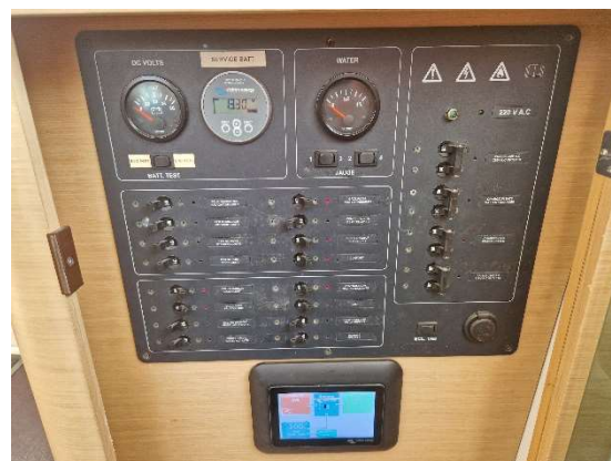
main switchboard with generator controller
