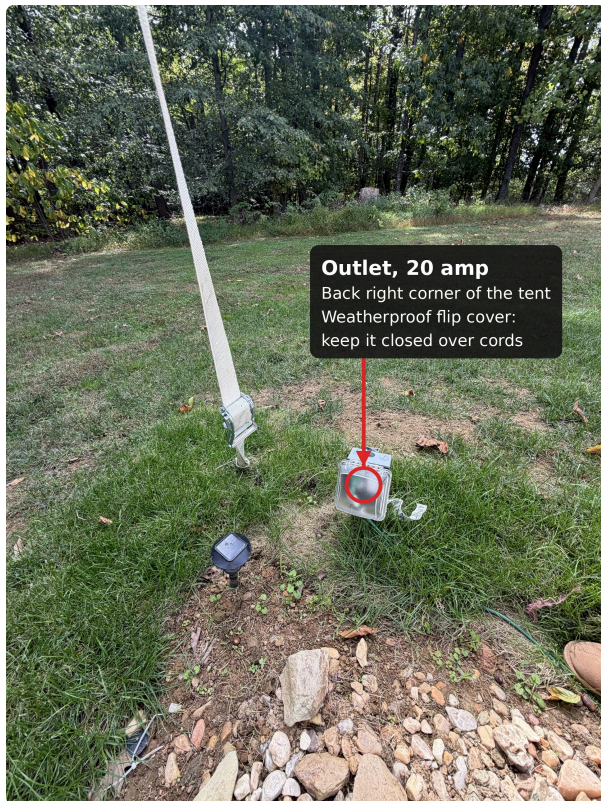
Back right outlet post.
