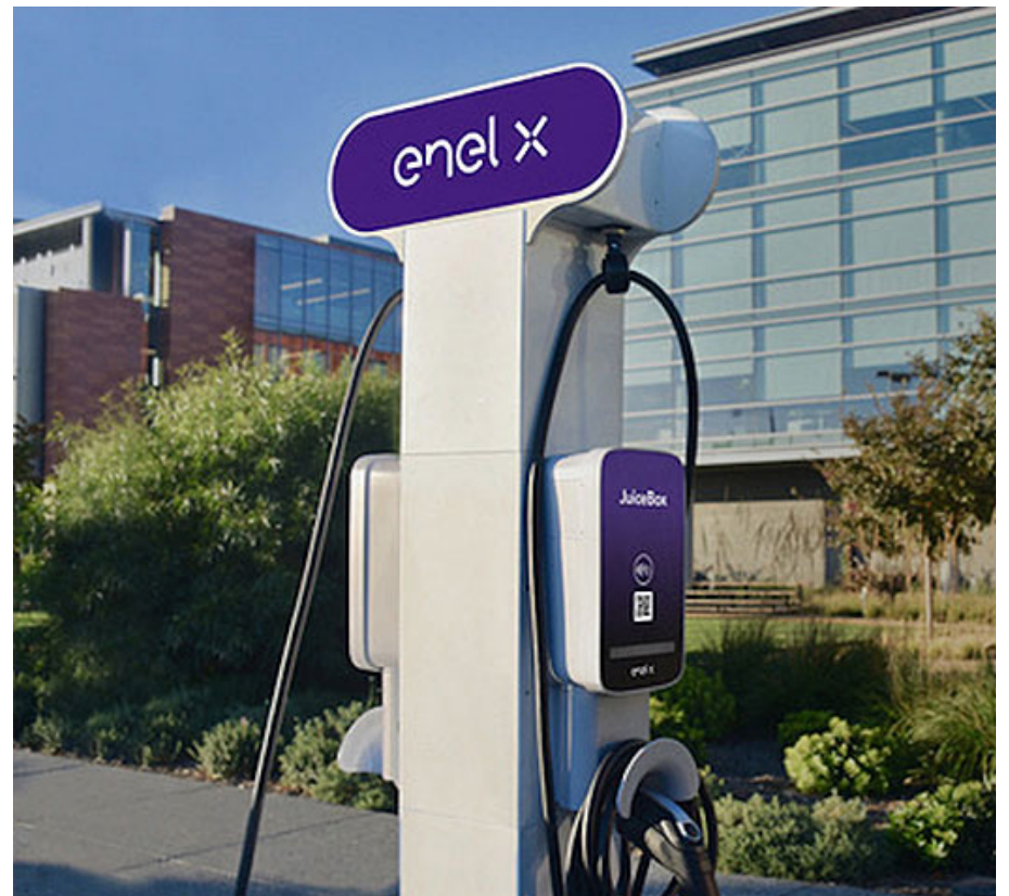
An Enel X JuiceBox Pro EV charger
