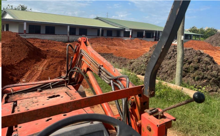
Filling in front of the school as part of the flood protection.
