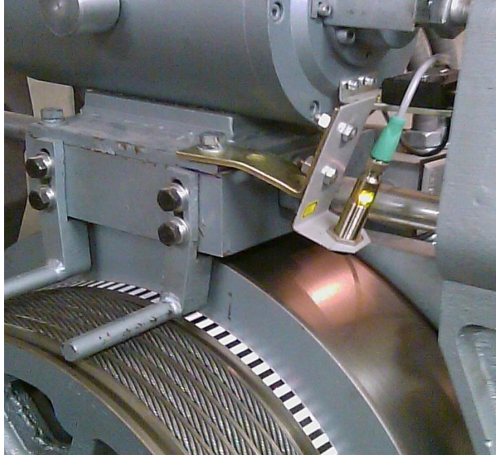
Figure 10: Installed ETSD Tape & Speed Sensor
