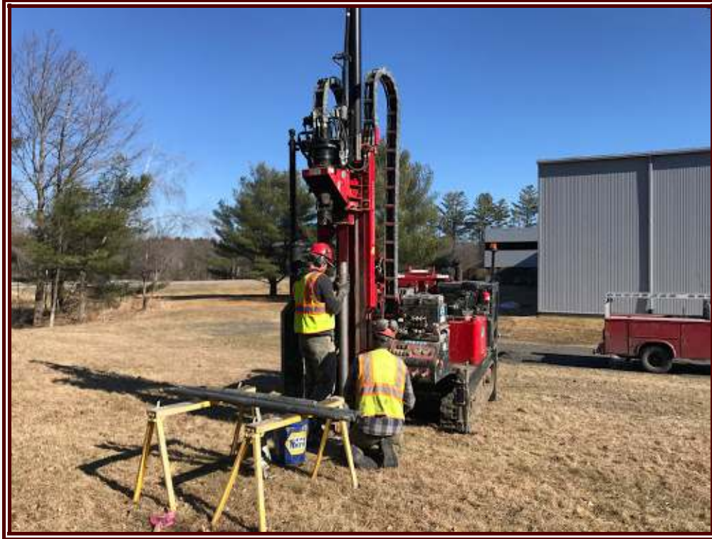
Figure 16 With the aid of a machine it is possible to bore in one day as many as 12 soil cores down to depths of 15 feet, i.e. up to 180 feet of borings per day.
