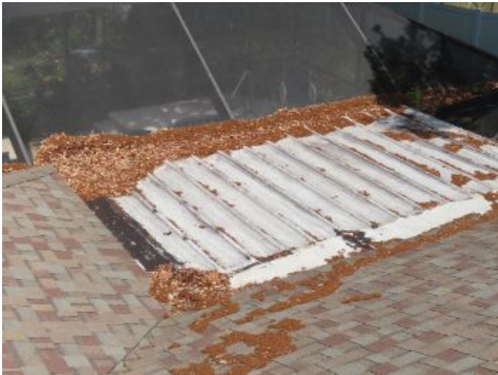
Leave build-up on roof
