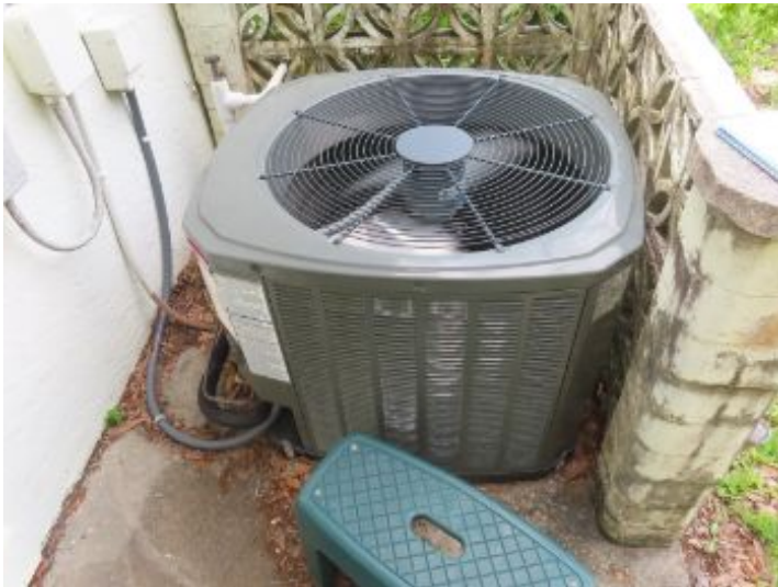
Electric, HVAC, Plumbing HVAC Unit
