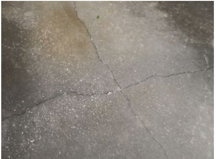
Cracked Concrete at Driveway
