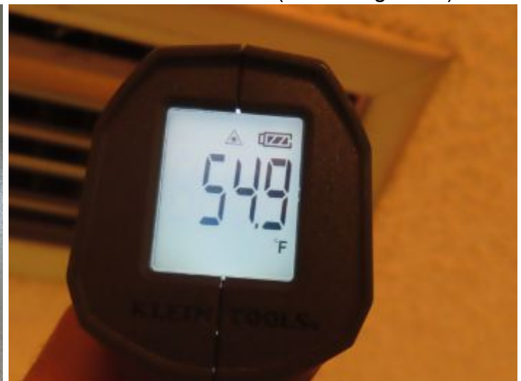
Electric, HVAC, Plumbing HVAC Unit
