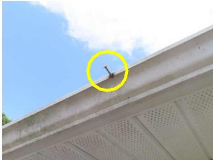
Loose gutter spikes
