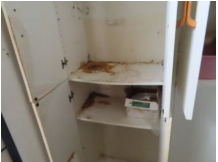
Damaged garage cabinetry
