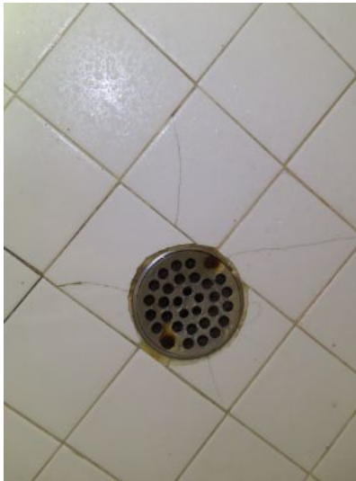
Cracked tile at shower floor
