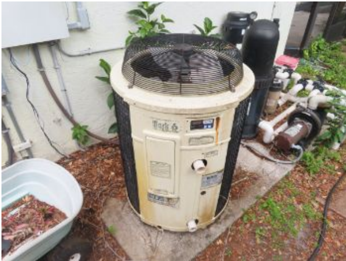
Pool heater - Not plumbed to pool - Assumed to not be in working order
