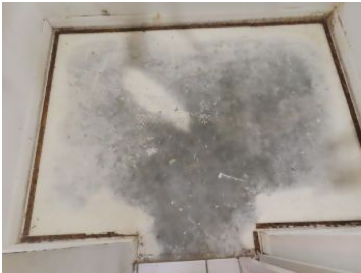
Closet carpet missing
