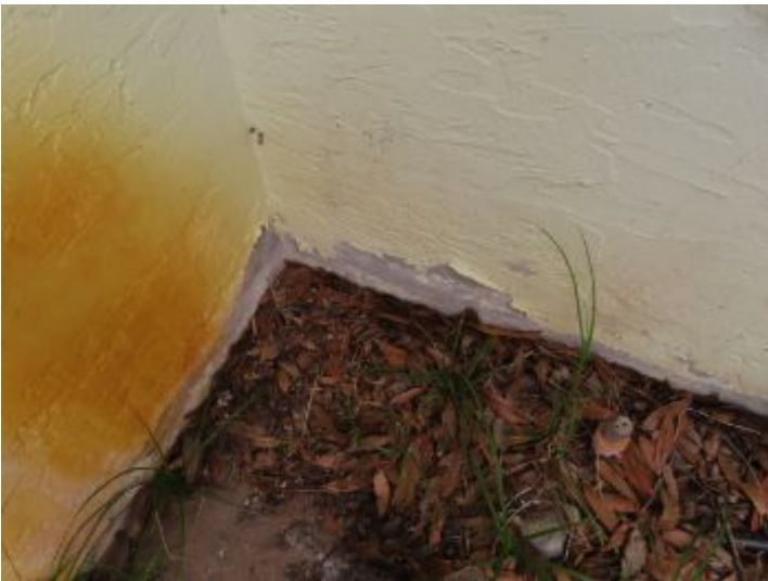
Peeling wall paint
