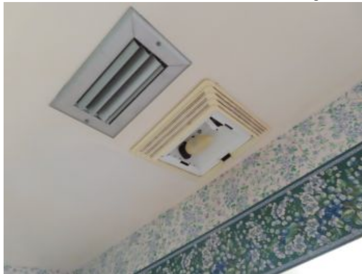
Light cover missing
