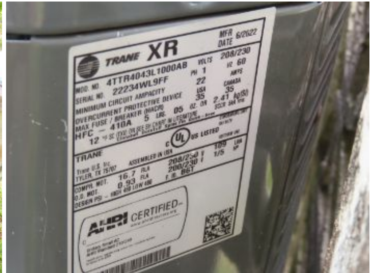
Electric, HVAC, Plumbing HVAC Unit
