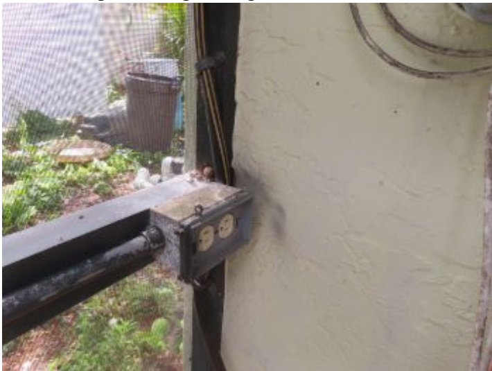
Damaged exterior electrical
