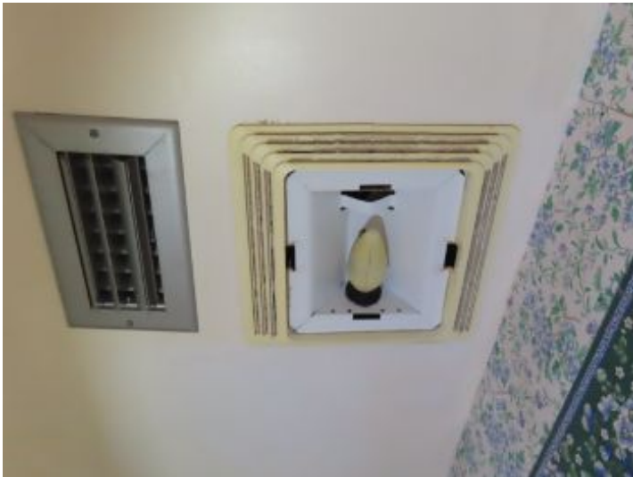
Cover missing at master bath
