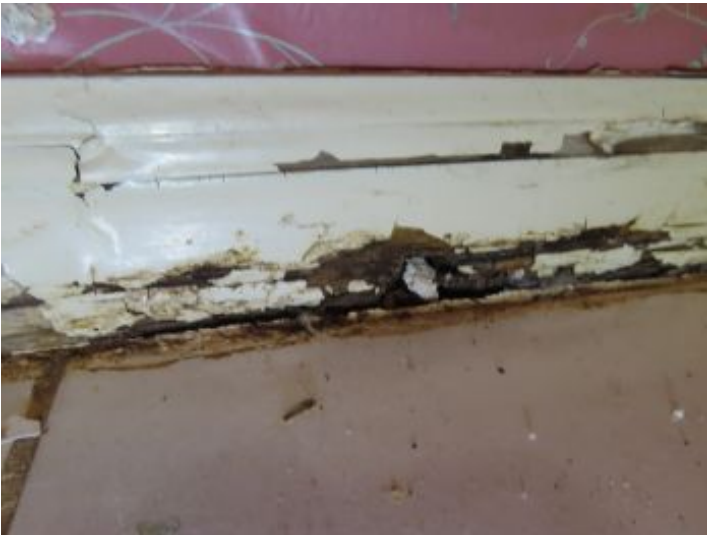
Damaged baseboard - Appears to be water damage
