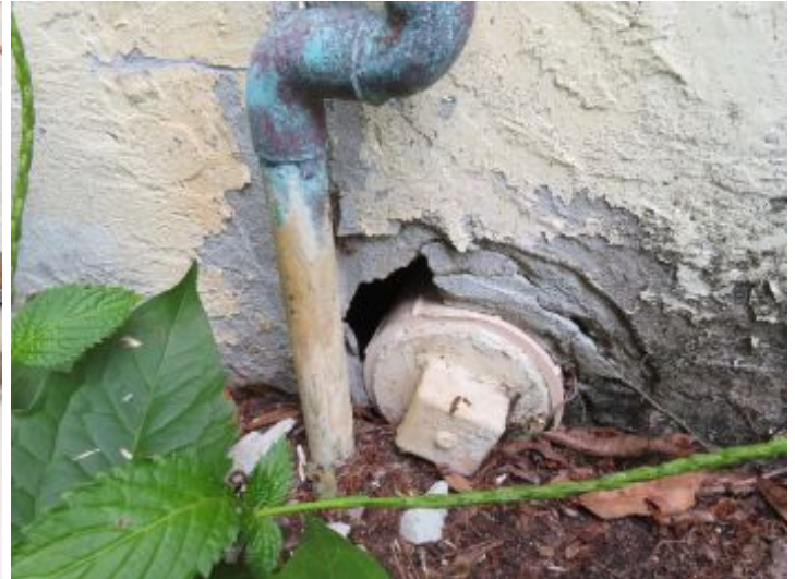
Stucco patch needed at clean out
