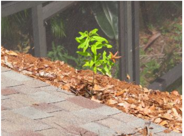
Leave build-up on roof
