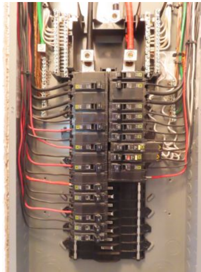
Electric, HVAC, Plumbing Electrical Panel
