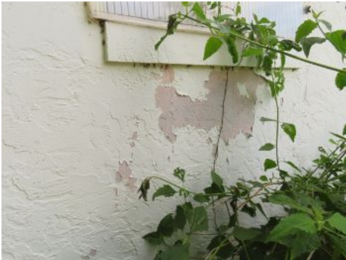
Peeling wall paint
