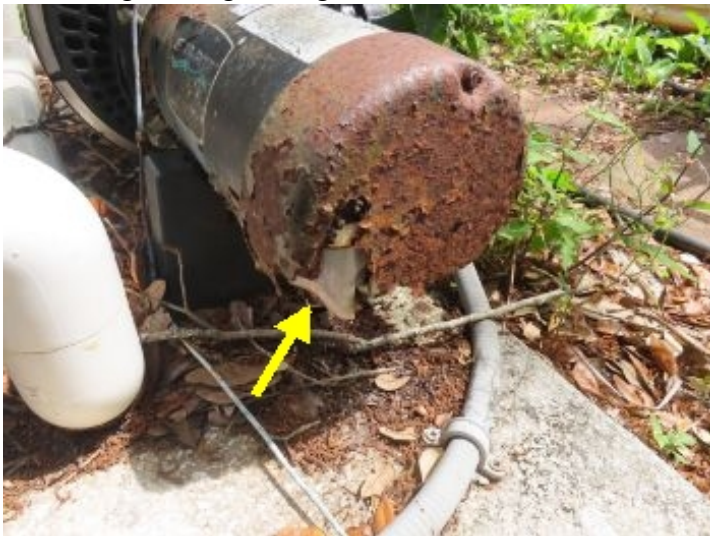
Rusted spa pump - Cannot confirm if pump is in working order
