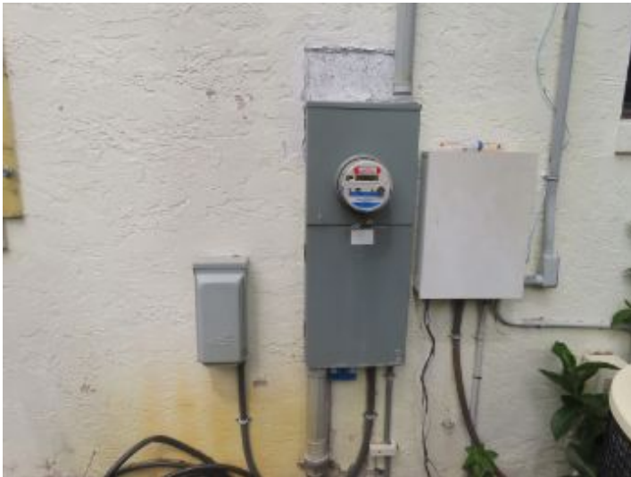
Electric, HVAC, Plumbing Electrical Panel
