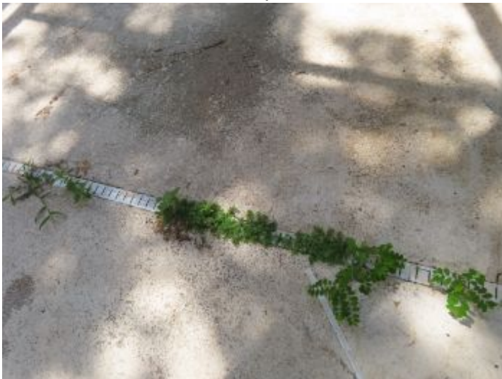
Vegetation growing out of deco drain
