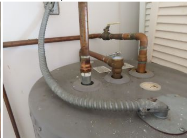
Water heater TPR valve
