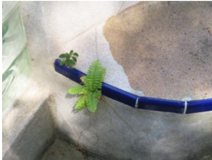
Organics growing out of hairline cracks
