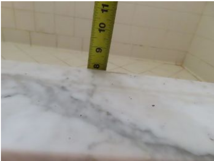
Large step down into shower - Trip hazard
