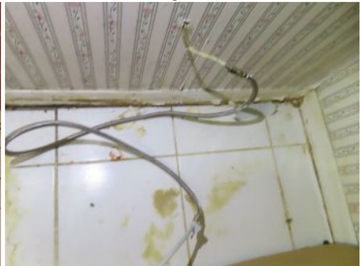
Area behind refrigerator showing water line
