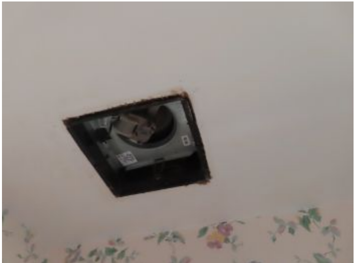
Light cover missing
