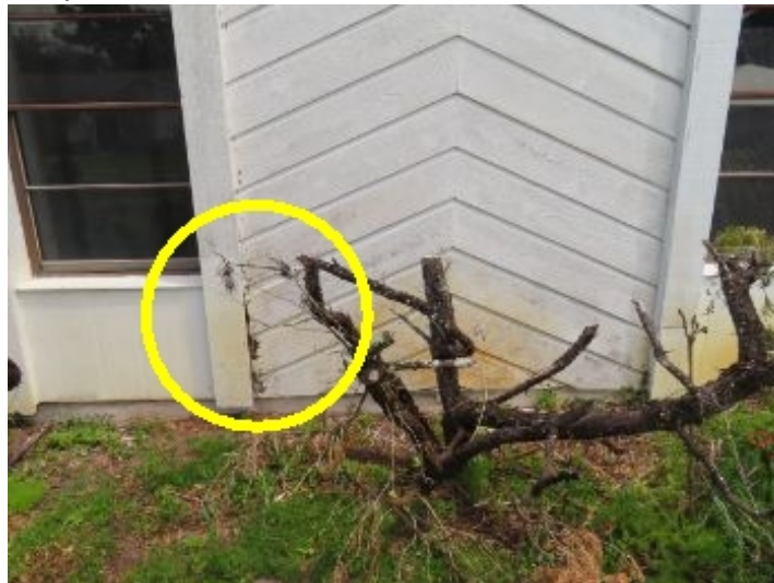
Wood rot at front Chevron
