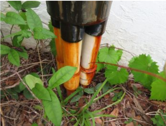
Irrigation indexing valve- Leaking at plumbing fitting
