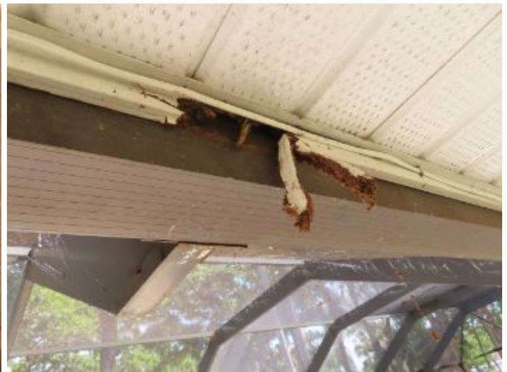
Wood rot at rear fascia behind screen super gutter
