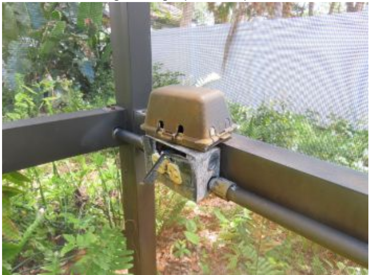
Damaged exterior electrical
