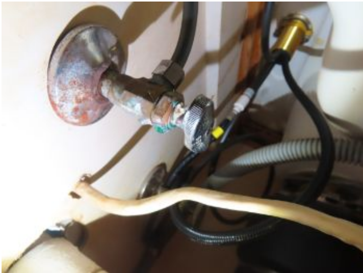
Corroded water shutoff valves at kitchen sink vanity
