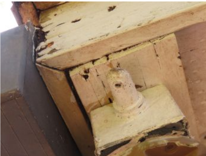
Wood rot at left rear corner fascia
