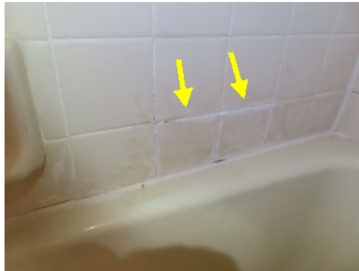
Possible tile repair area
