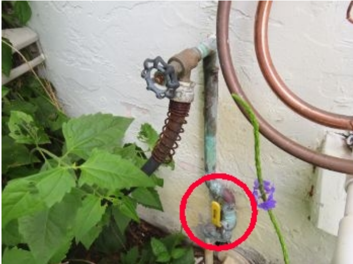
Main water shutoff valve - Left elevation
