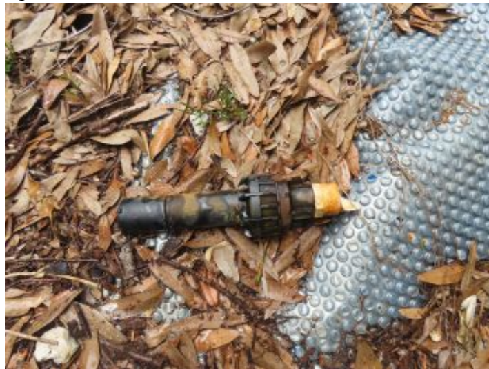
Damaged irrigation head laying on ground
