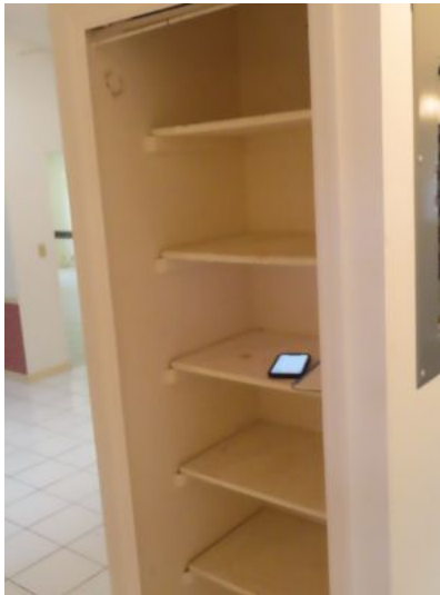
Closet missing doors
