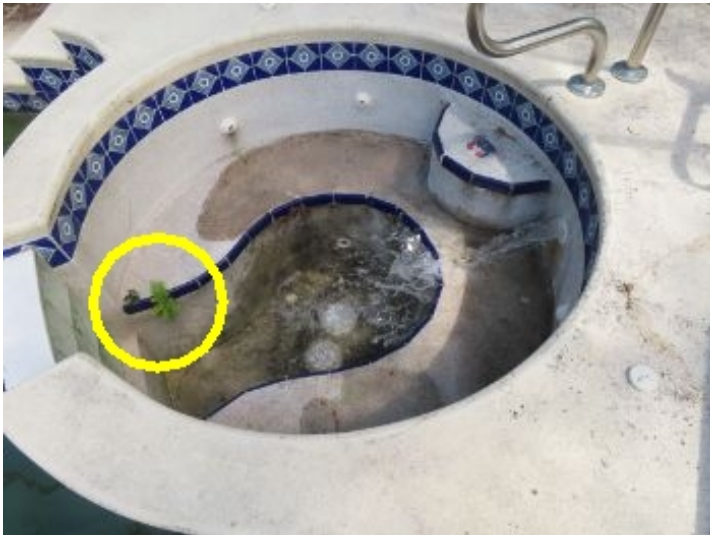
Organics growing out of hairline cracks
