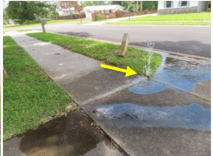
Damaged irrigation head
