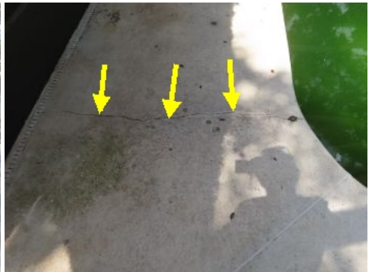
Concrete crack at pool deck
