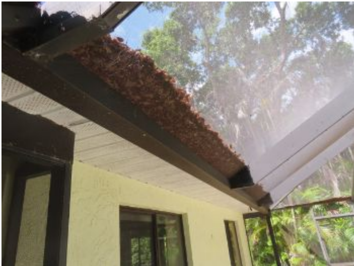
Debris build-up on screen
