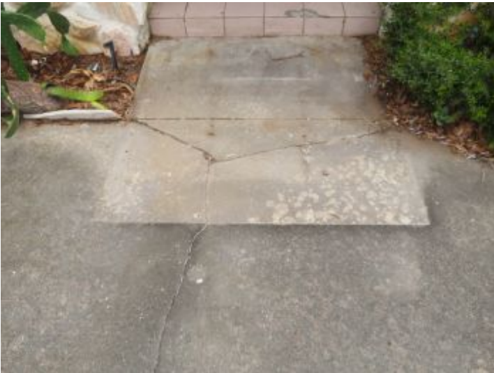
Cracked Concrete at Driveway
