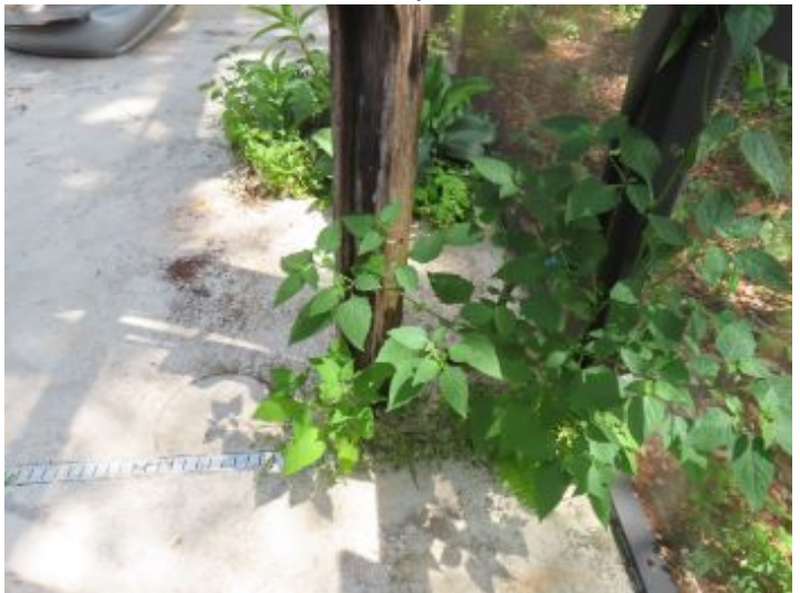
Weeds growing up out of pool deck
