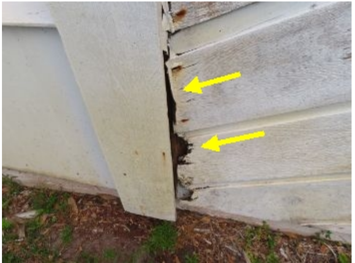
Wood rot at front chevron
