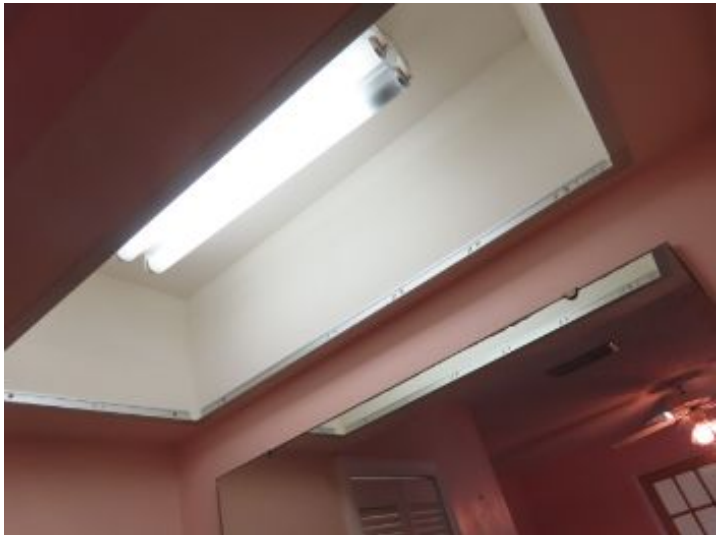
Light cover missing
