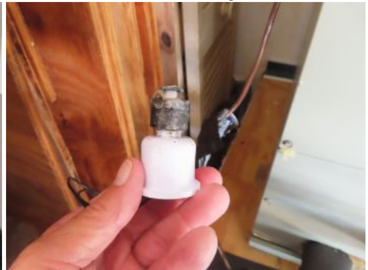
AHU Safe-T-Switch (in working order)
