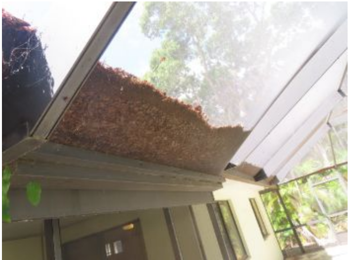
Debris build-up on screen
