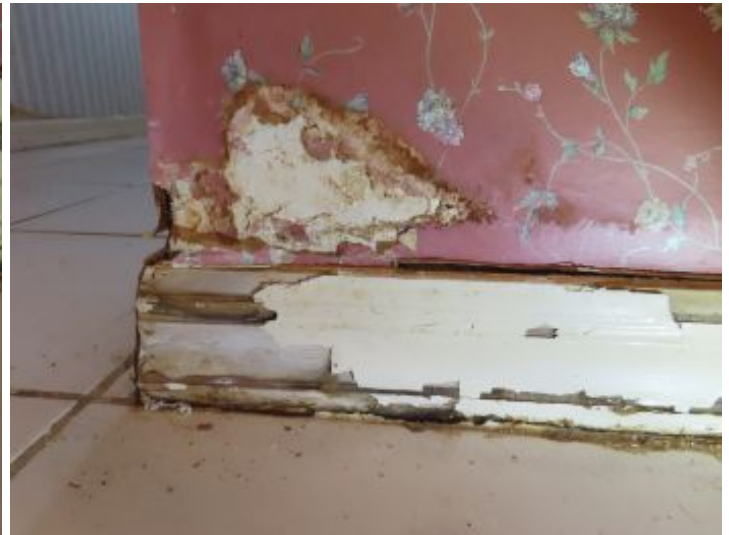
Damaged baseboard - Backs up to kitchen refrigerator
