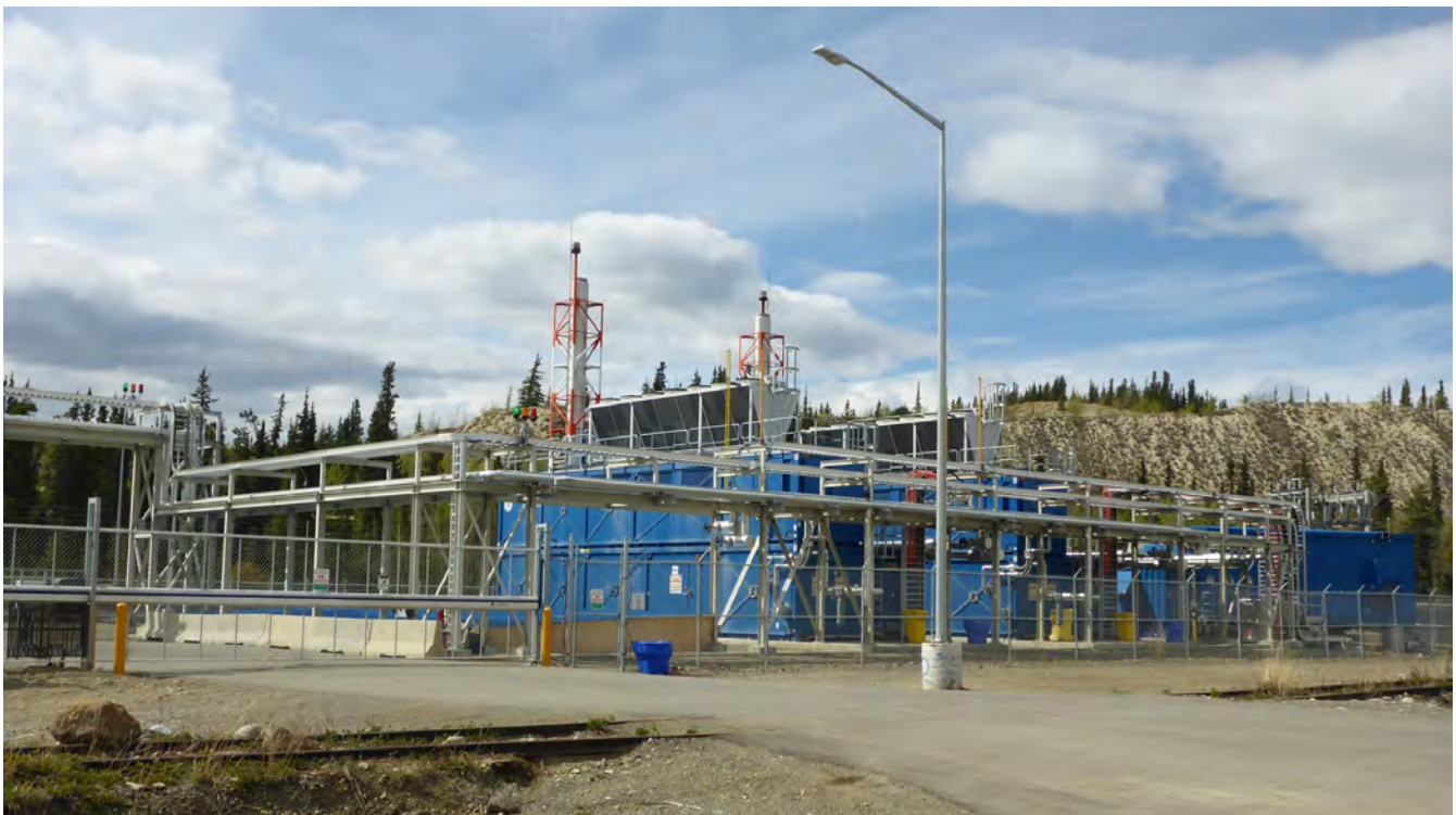
YEC's Liquefied Natural Gas (LNG) electrical generating plant
