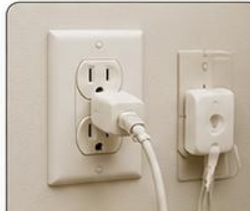
ELECTRICAL OUTLETS Use safety covers.
