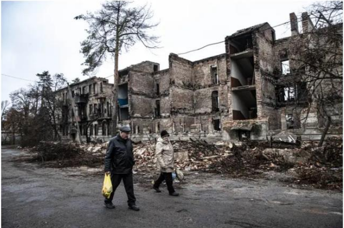
Destroyed apartments in Lyman after the Ukrainian city was recaptured from Russia forces in November 2022. Metin Aktas/Anadolu Agency via Getty Images
