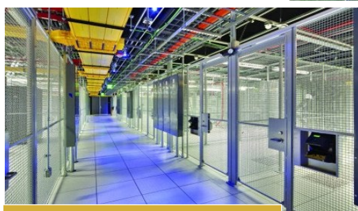
Colocation, Equinix, Dallas, USA
