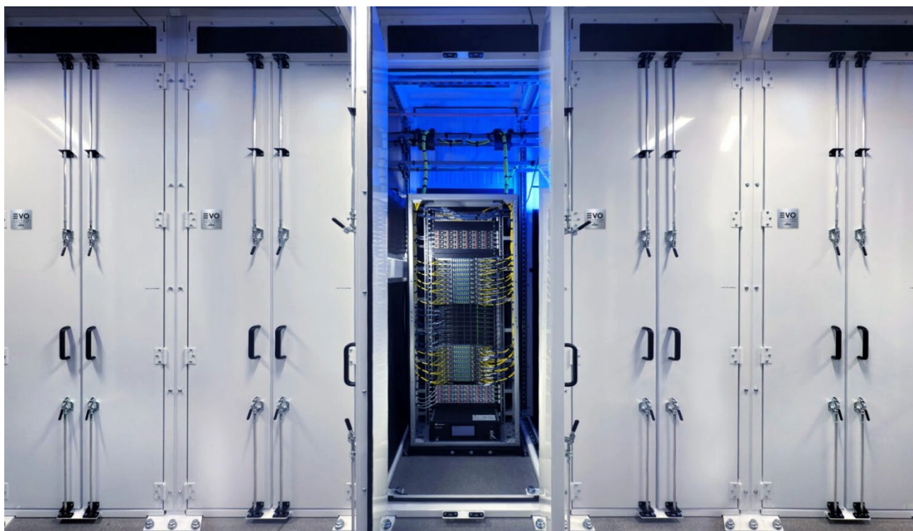
NVIDIA GB300 NVL72 rack, deployed by CoreWeave in a Switch Data Centre, USA The NVIDIA Vera Rubin GB300 NVL72 features a fully liquid-cooled, rack-scale architecture that integrates 72 NVIDIA Blackwell Ultra GPUs and 36 Arm®-based NVIDIA Grace™ CPUs into a single platform. Price per rack is between US$4-US$6 million
