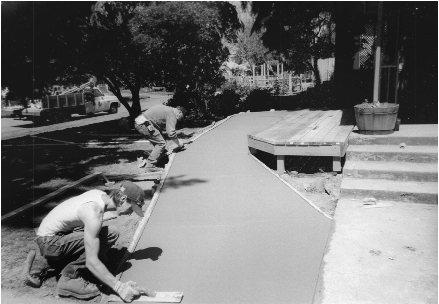
Workers are troweling the concrete ramp to make my new home accessible.
