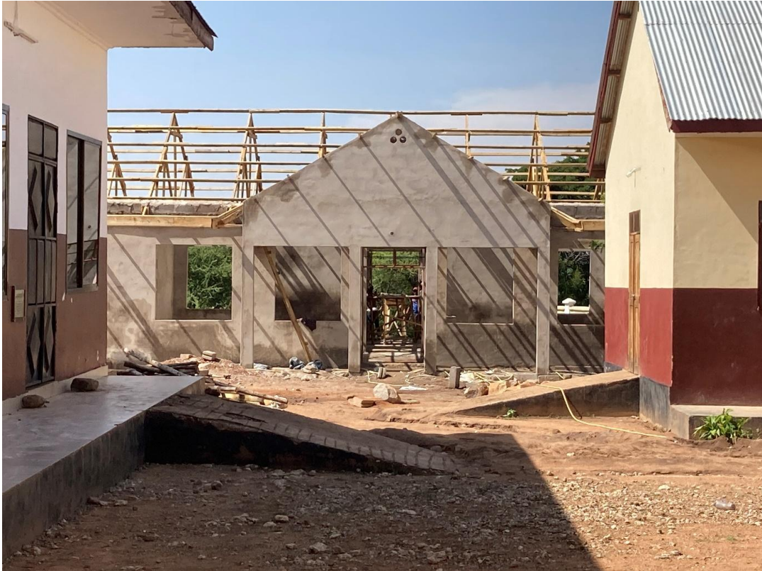
Annex A New hostel under construction for girls who survived the fire
