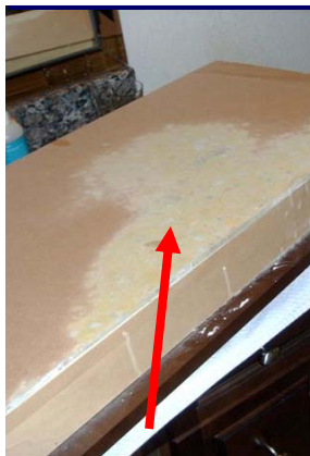
Mold growth on back of medicine cabinet, third floor bathroom
