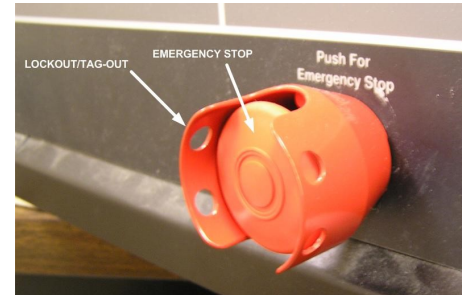
Figure 4: Disconnect requirements for a non-paralleled generator set can often be met using an emergency stop switch with lock-out/tag-out provisions.
